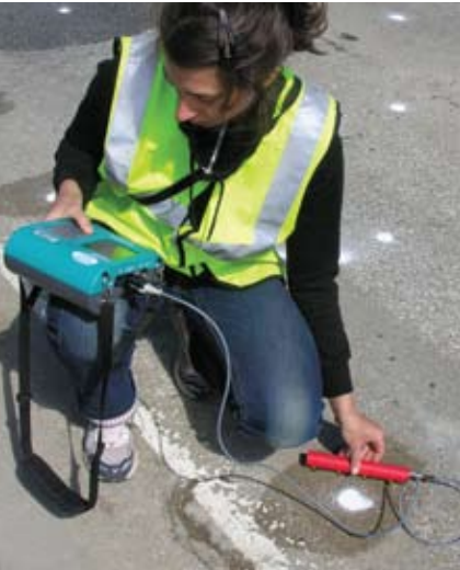
Sabine Kruschwitz, a visiting researcher from Germany, tests electrical resistivity of the concrete, an indicator that can be linked to rate of corrosion. Using multiple NDE tests helps give the most thorough "picture" possible.
