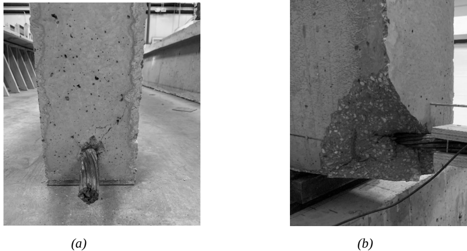
Figure 4-14 Live end surface cracking on beam 1 (a), and beam 3 (b)
