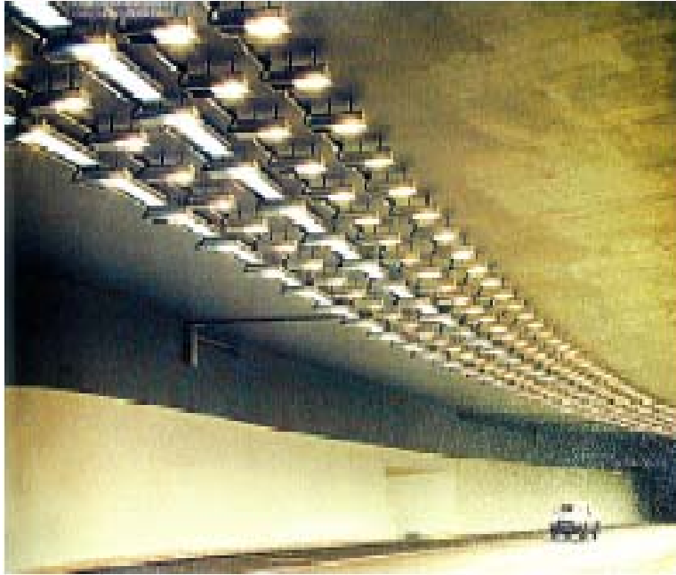
Figure 43 : Tunnel Induction Lighting
