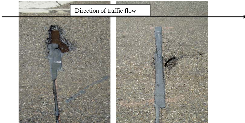
Figure 76 Failure of sensor assemblies; outside of lane (left) and inside of lane (right).
