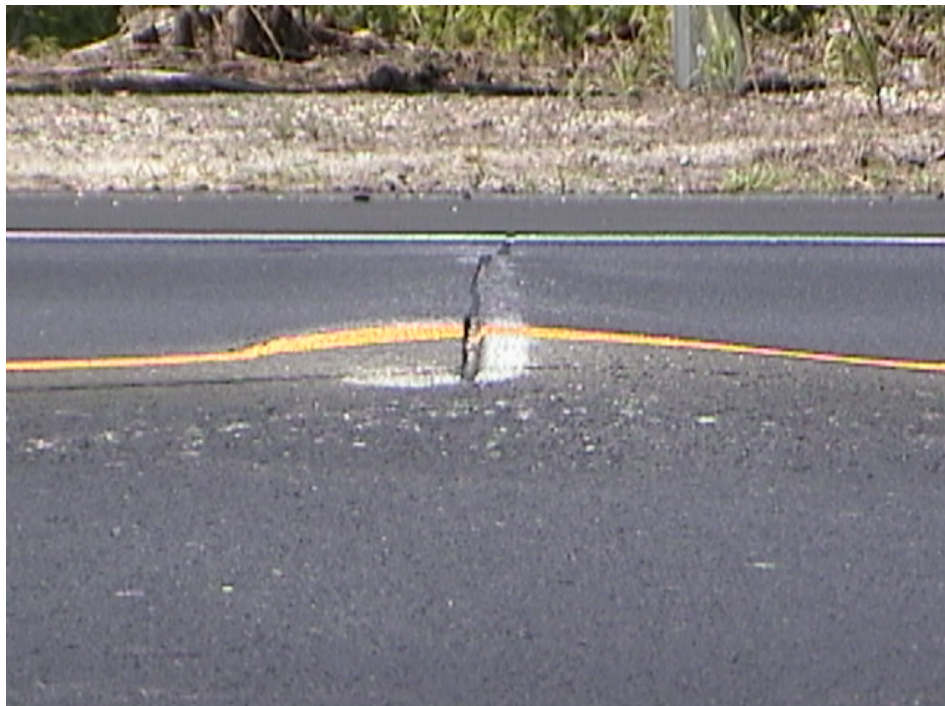
Figure 6 – HMA Overlay on Route 34 (Picture taken from Northbound Side showing the joint was only sawed and sealed on the Southbound Side)
