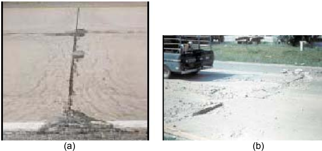
Figure 7 – (a) Durability Cracking (D-Cracking) of PCC Pavement; (b) Blow-up of PCC Pavement
