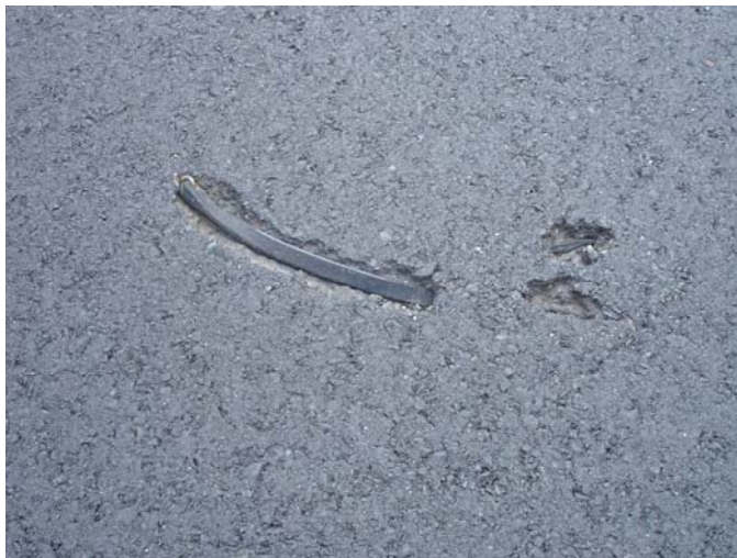
Figure 49 – Rubber Cord Paved into Pavement Surface of Rt 202S in New Jersey
