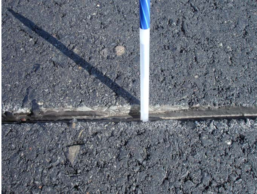
Figure 51 – Poor Sealing of Sawed Joints from Rt 202S in New Jersey
