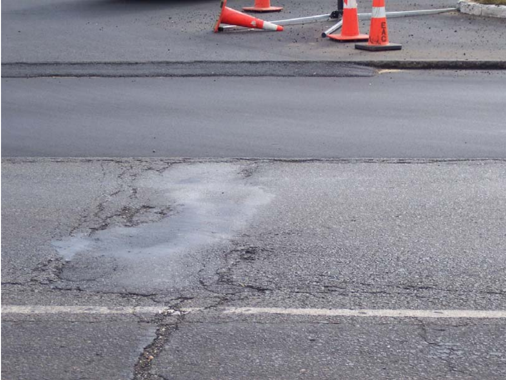
Figure 27 – Photo of Reflective Crack Relief Interlayer (RCRI) Mix, shown in far lane, and Existing HMA Patch Over Deteriorated Reflective Crack
