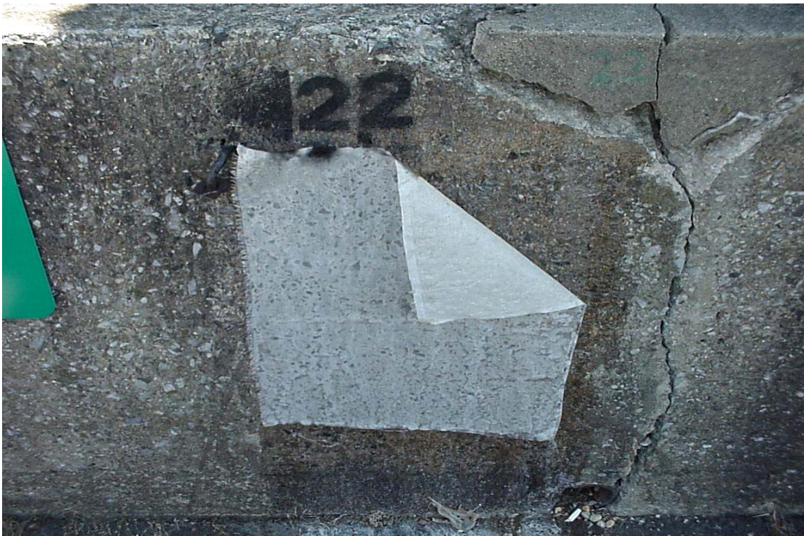
Figure 4.6: Delamination of Tyfo S® Composite under Wet Conditions on the Day Three
