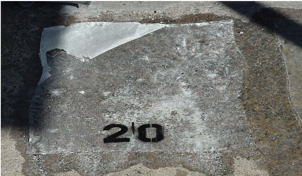
Figure 4.4: Delaminating Tyfo S® Composite under Wet Conditions Three Days after Laminating
