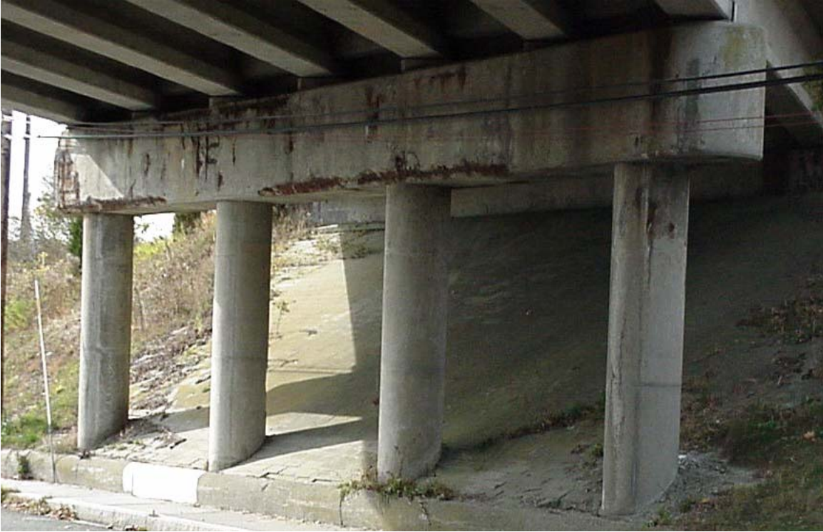
Figure 2.2 : Deteriorated Pier Cap of Salt Pond Road Bridge
