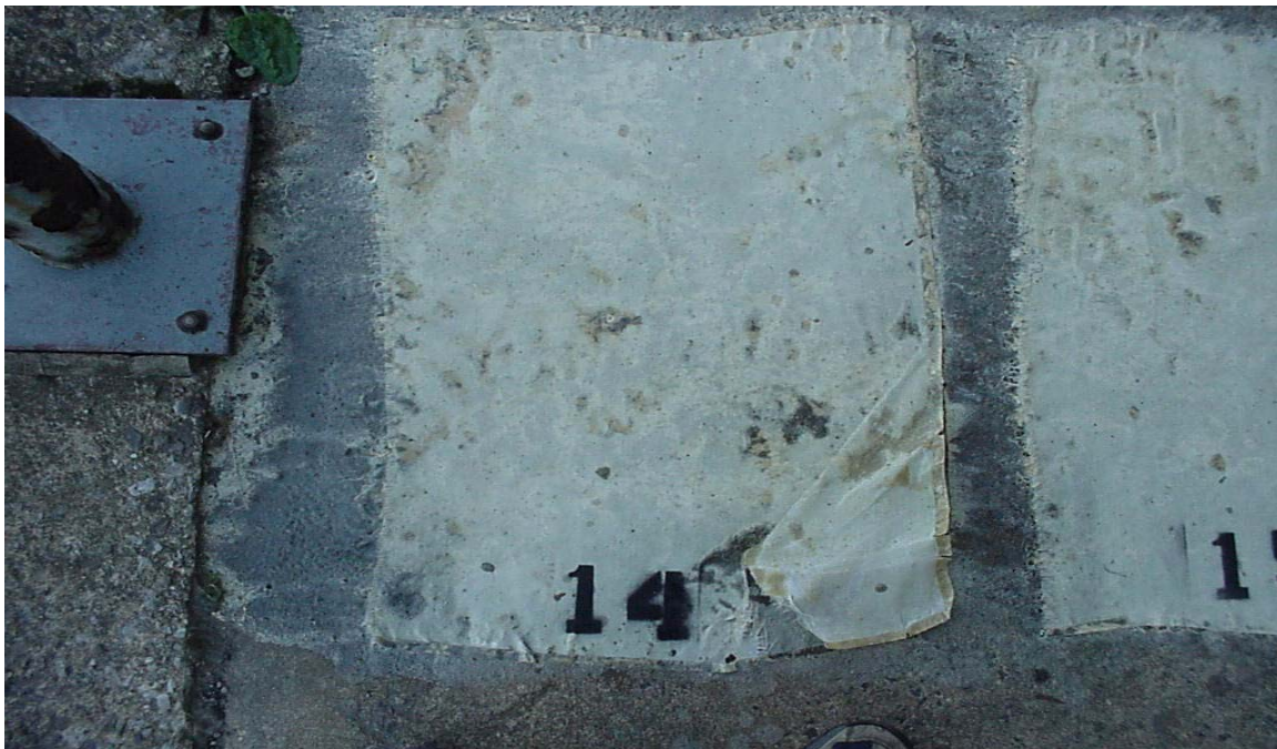
Figure 4.2: Tyfo S ® Composite Delaminating Under Wet Conditions 2 Days after Laminating
