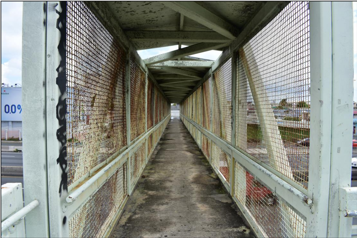
Figure 6.40: Corrosion on the superstructure of PB 2683
