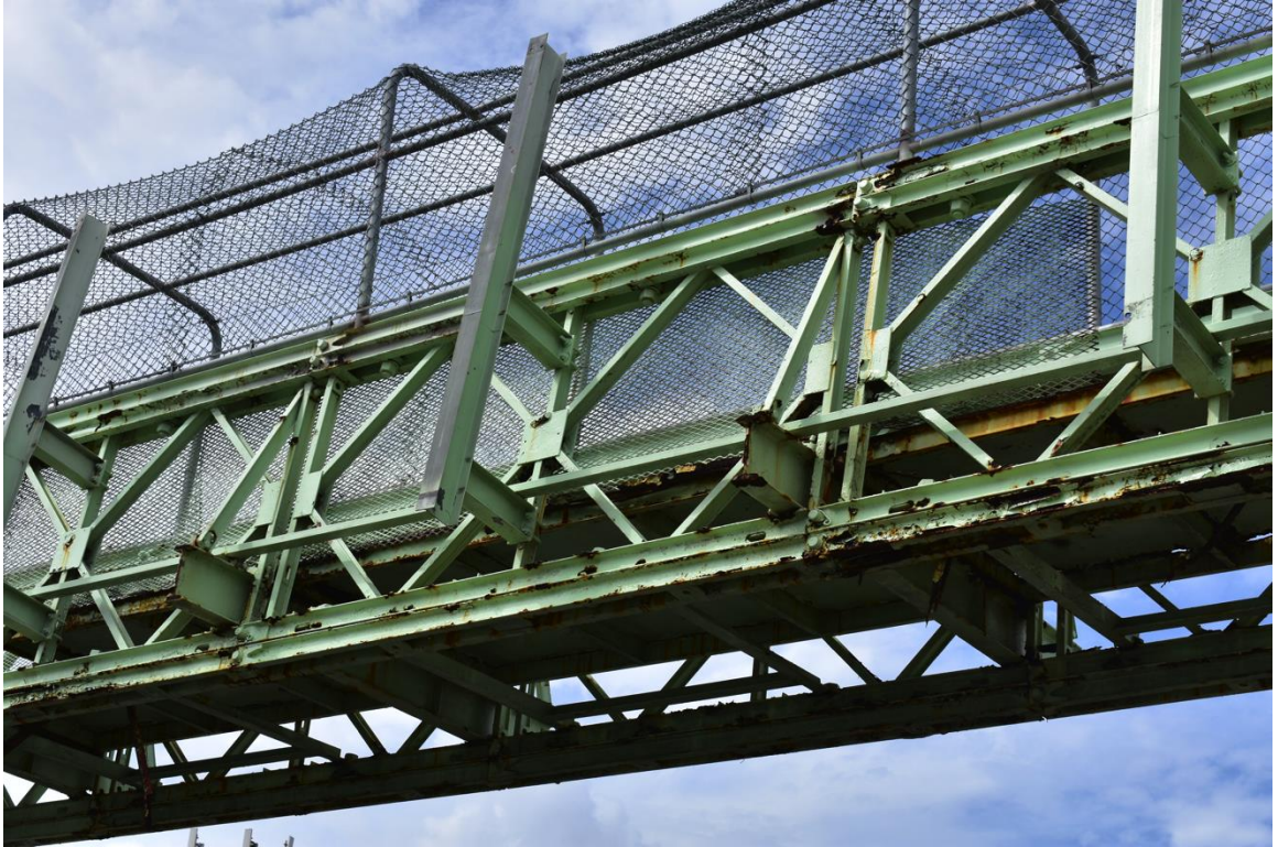
Figure 8.10: Signage Support Structure (2 of 3)
