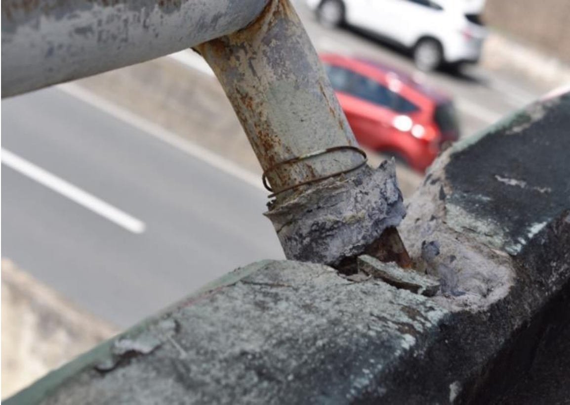
Figure 5.19: Detached handrail post
