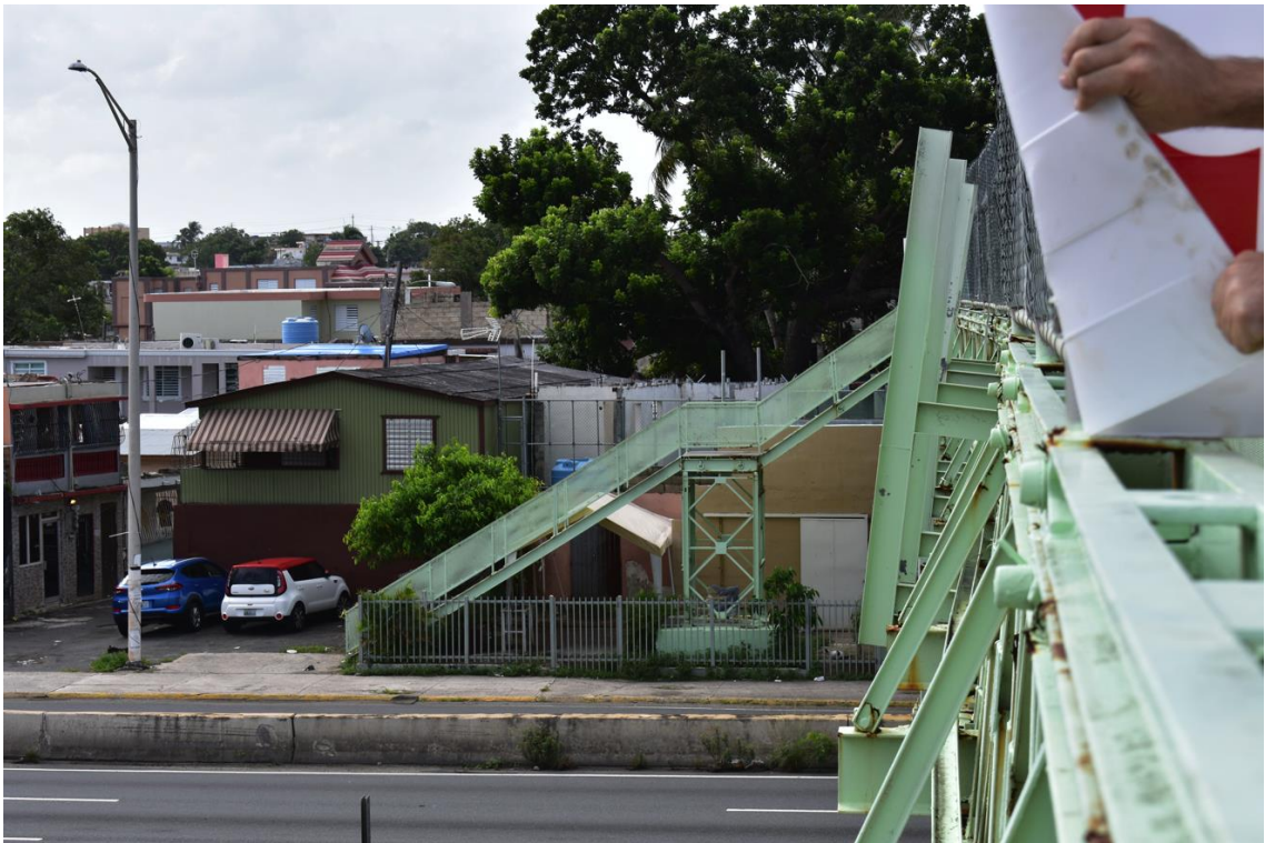
Figure 8.9: Signage Support Structure (1 of 3)
