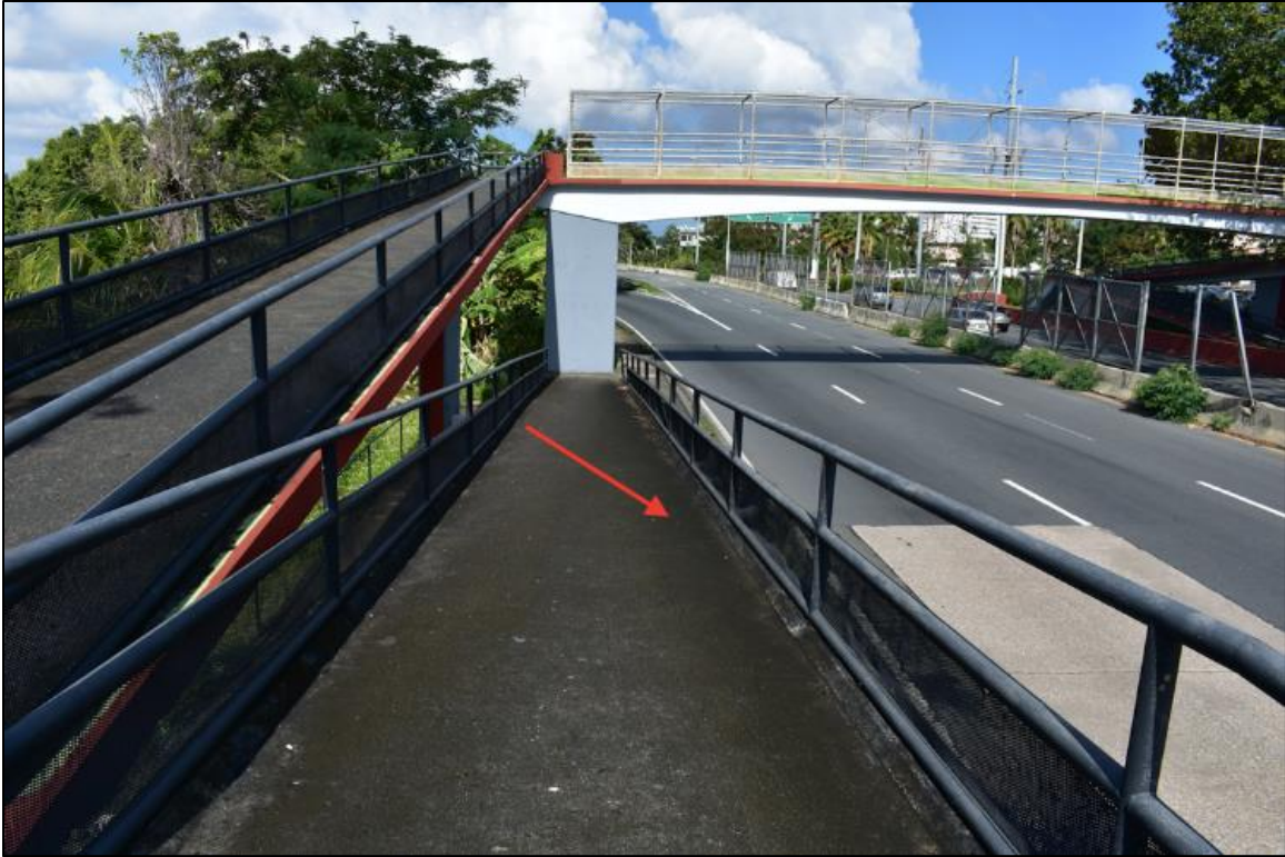
Figure 6.1: Mold and silt in the access ramps of PB 0626
