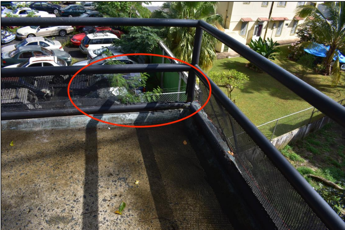
Figure 6.4: Missing section of safety meshing on PB 0626
