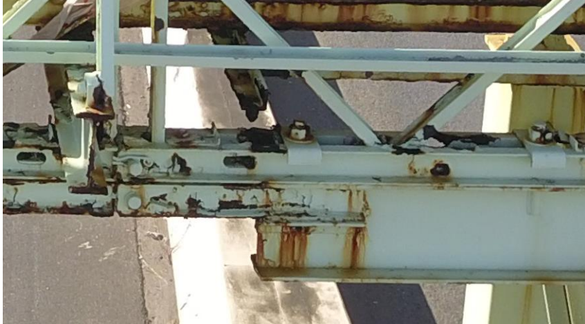
Figure 5.11: Corrosion in Truss Element (Example 2)
