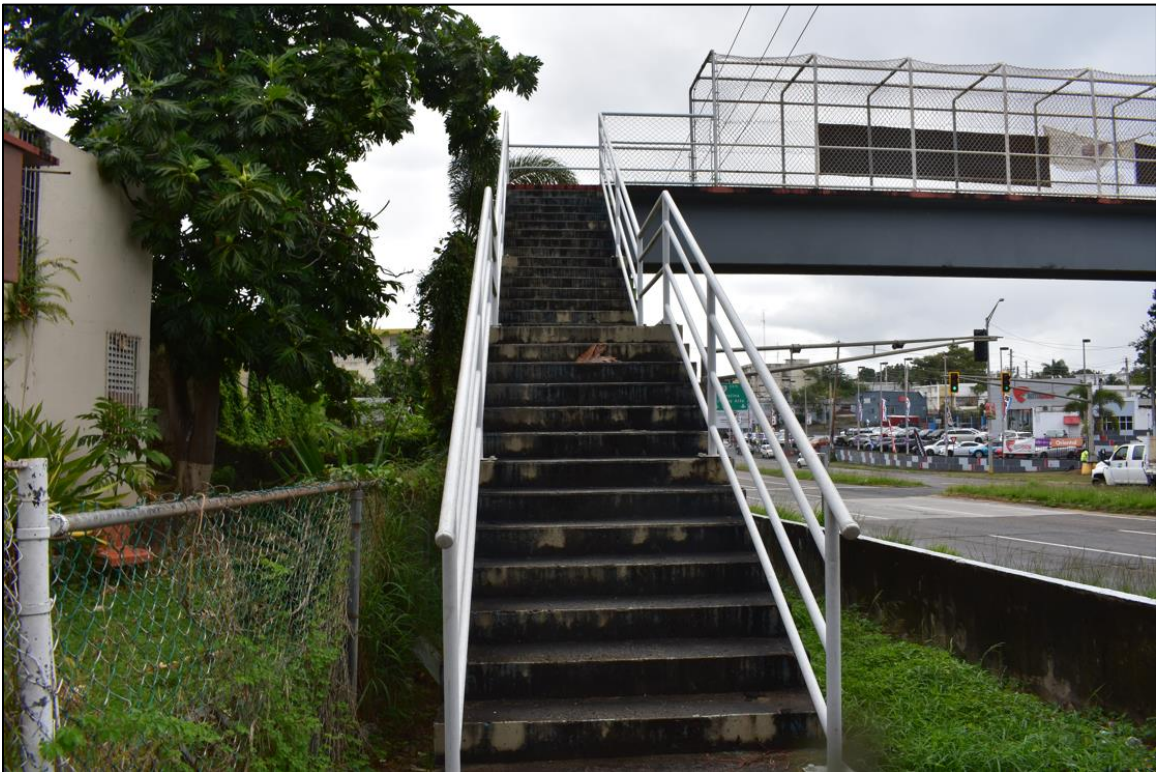
Figure 6.22: Mold and silt on stairway of PB 1736
