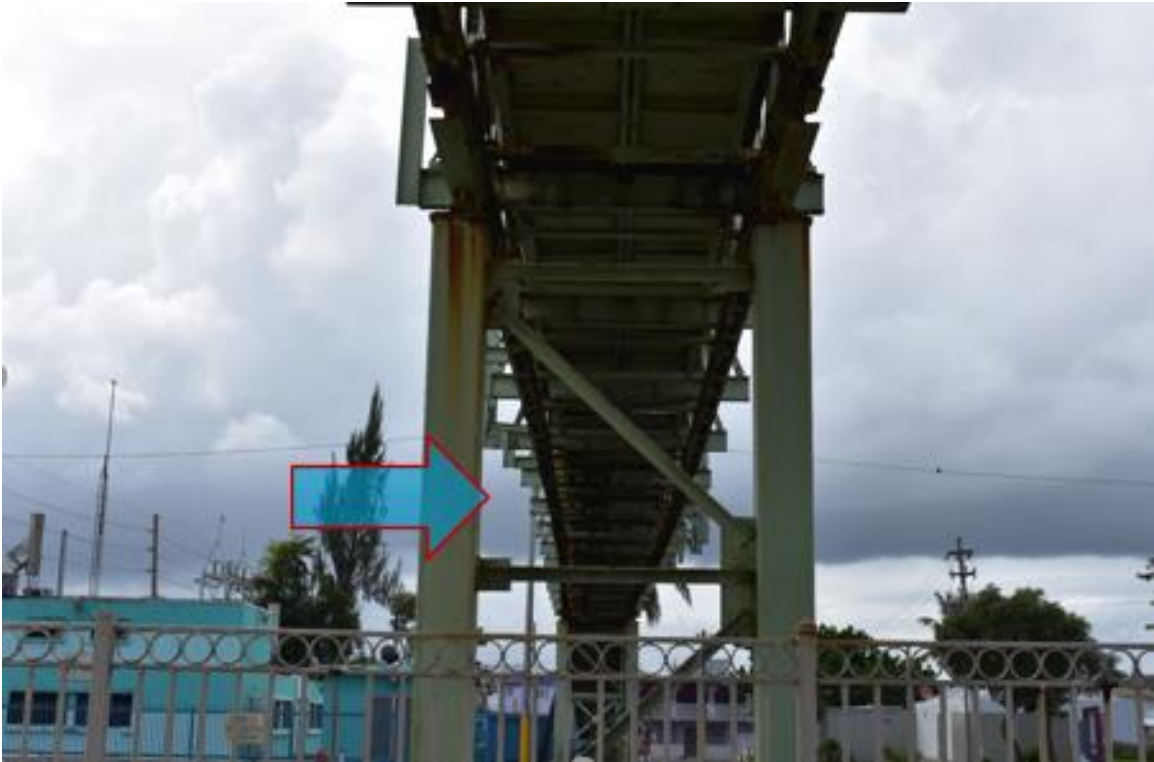
Figure 5.60: Underside of PB 1307 after Hurricane Maria (February 28, 2019)
