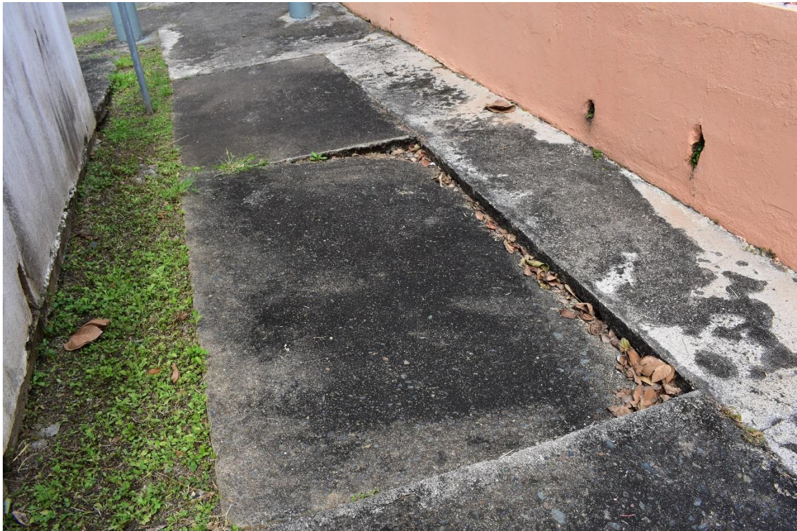
Figure 5.13: Sunk section of sidewalk
