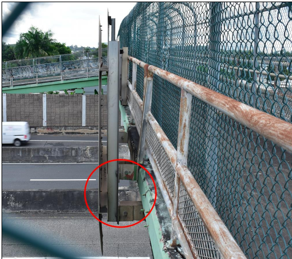
Figure 5.16: Traffic Signs partially detached from support
