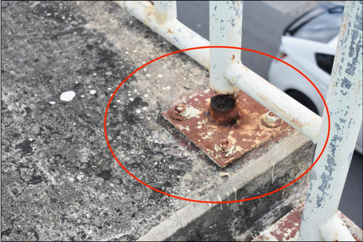
Figure 6.32: Corrosion of guardrail on PB 2087
