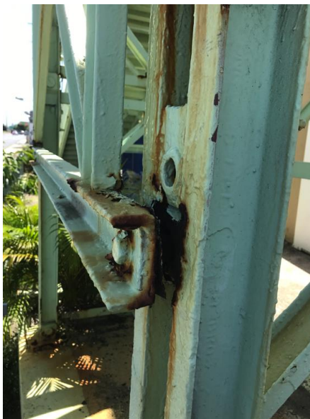
Figure 5.15: Loose Connection at Column Tower
