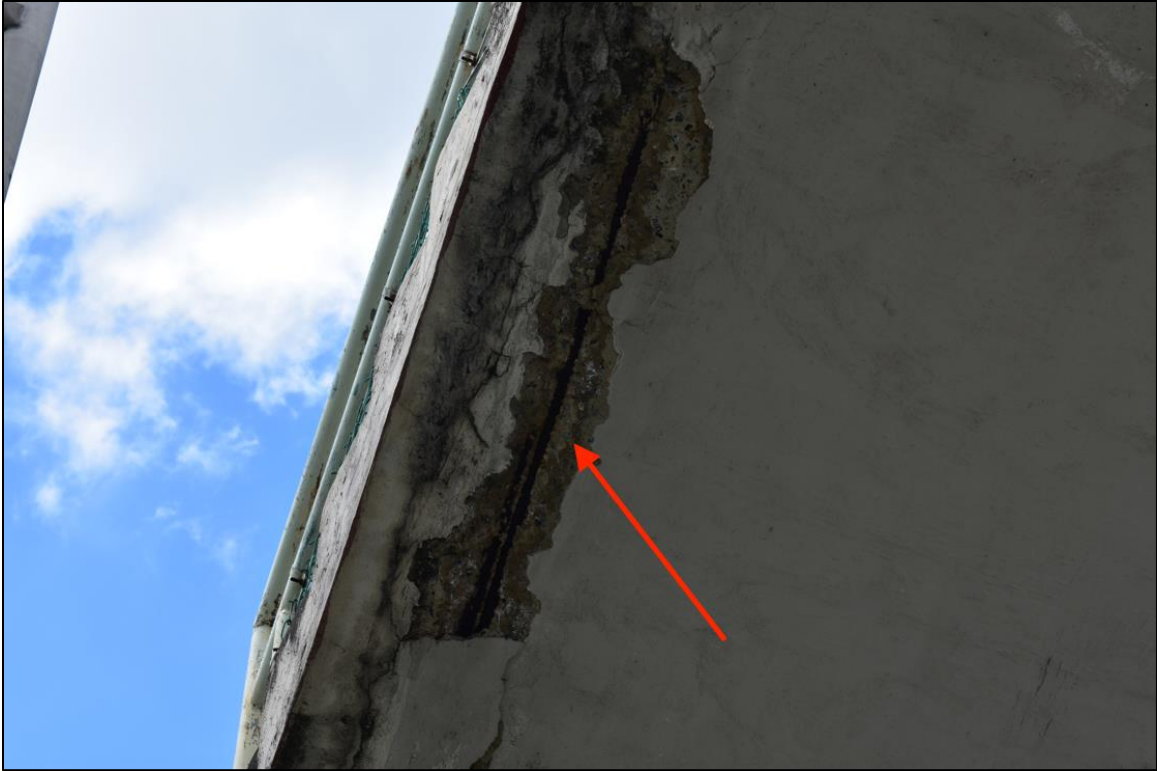
Figure 6.30: Exposed rebar on PB 2087
