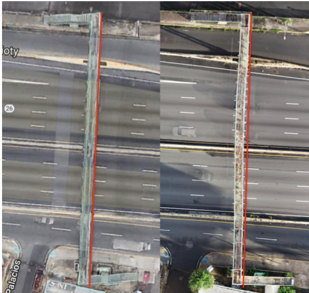
Figure 6.3: 2016 (Google Earth) and 2018 (Drone Survey) Bridge Geometry Comparison
