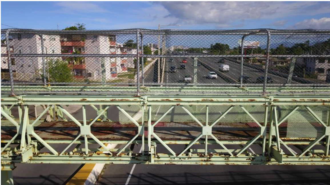
Figure 5.10: Corrosion in Truss Element (Example 1)
