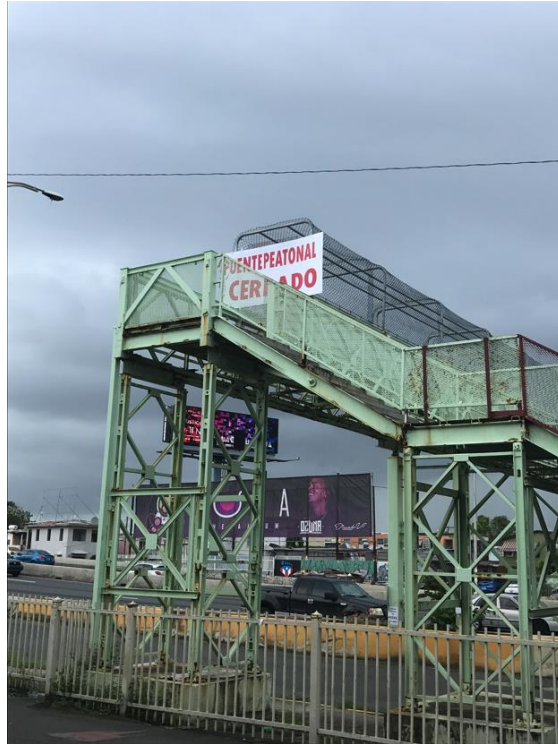
Figure 5.2: Sign Indicating Pedestrian Bridge is Closed
