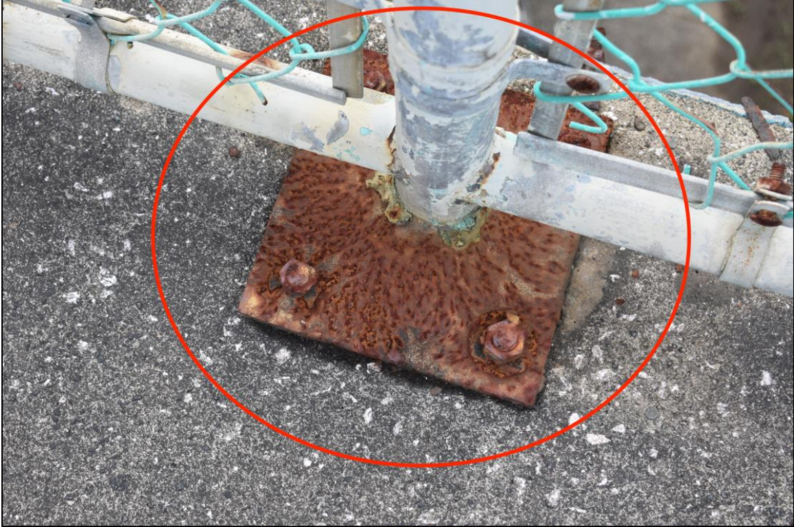
Figure 6.26: Corrosion of security fencing of PB 1743
