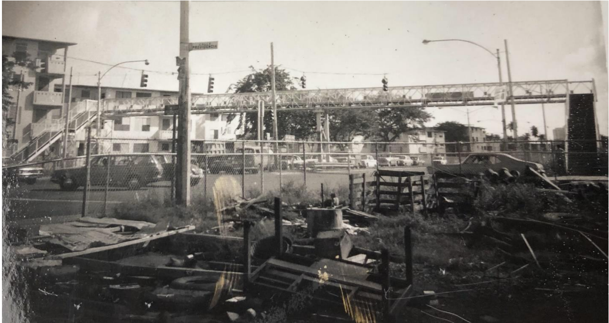
Figure 5.50: Phot of west side view of PB 1307 taken between 1968 and 1990 (Source: PRHTA)
