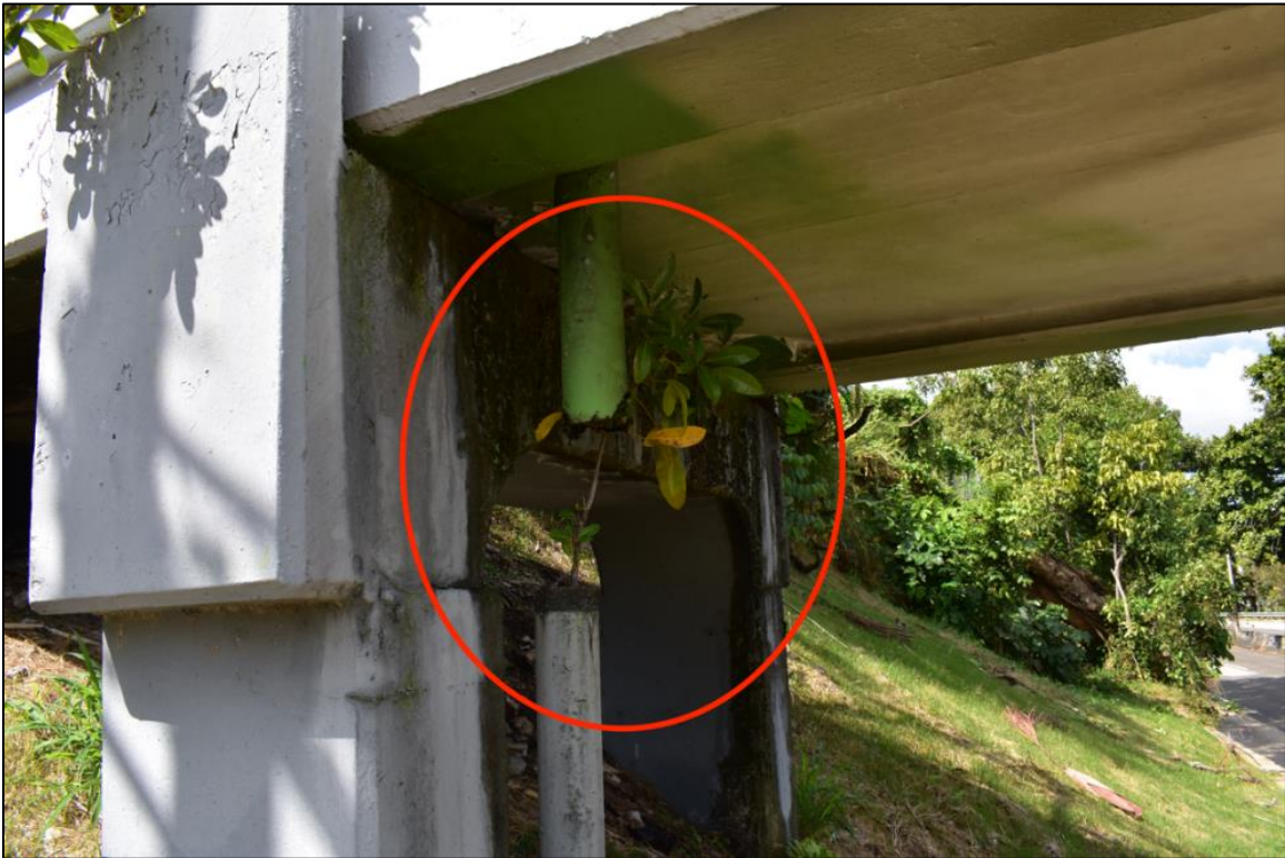
Figure 6.8: Broken drainpipe blocked with vegetation on PB 0748
