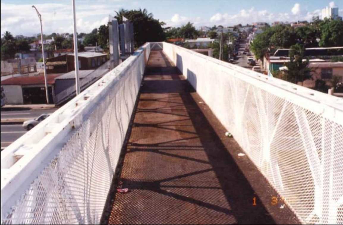
Figure 5.57: Deck of PB 1307 before Hurricane Maria (March 18, 1996) (Source: PRHTA)
