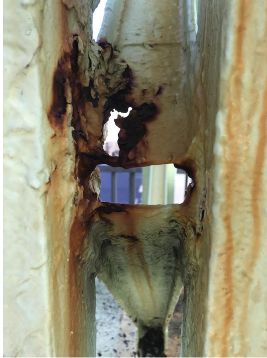
Figure 5.16: Section Loss due to Corrosion at Column Tower
