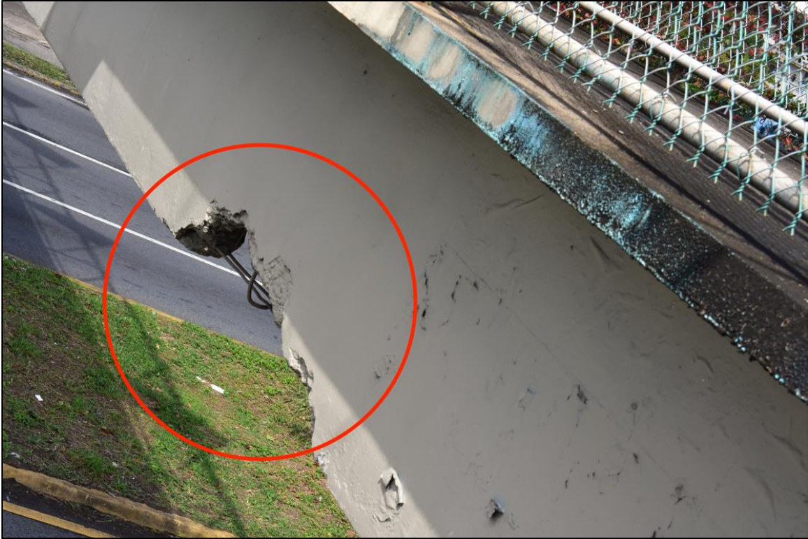
Figure 6.17: Exposed steel tendon on PB 1418
