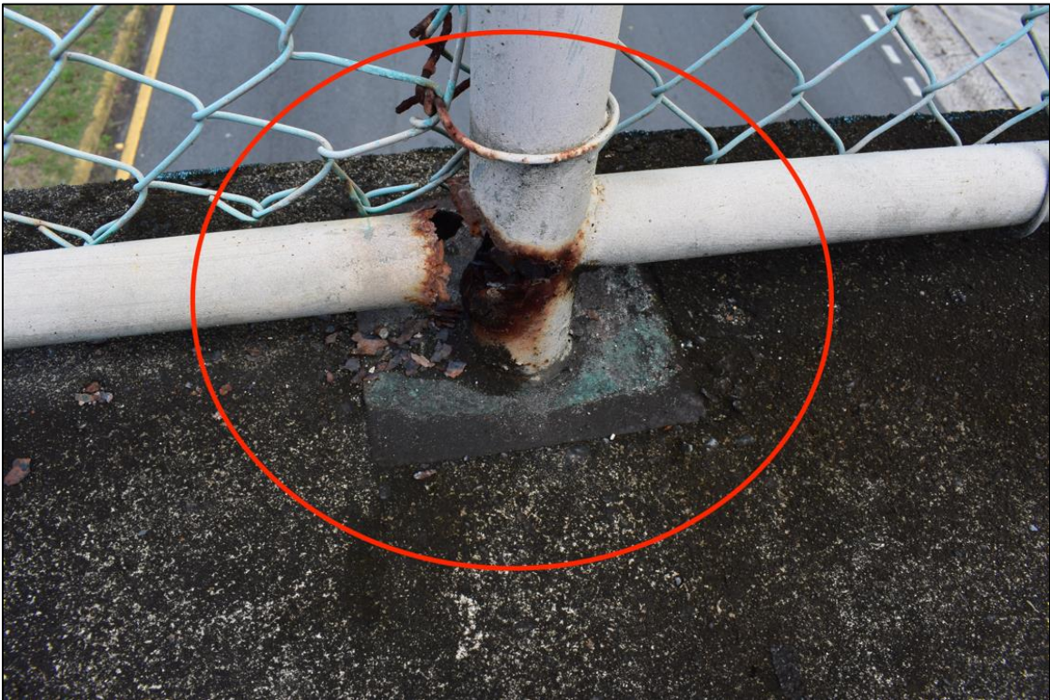
Figure 6.16: Corrosion on railing on PB 1418
