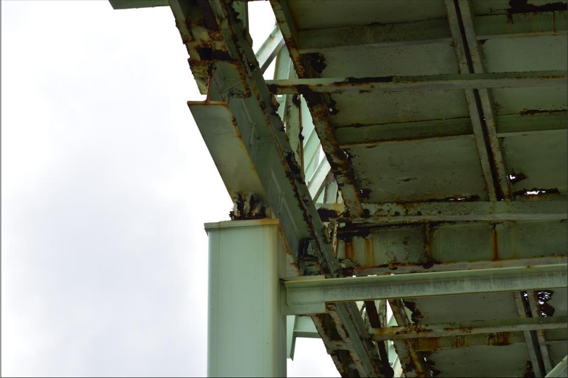
Figure 5.38: Some holes in the steel
