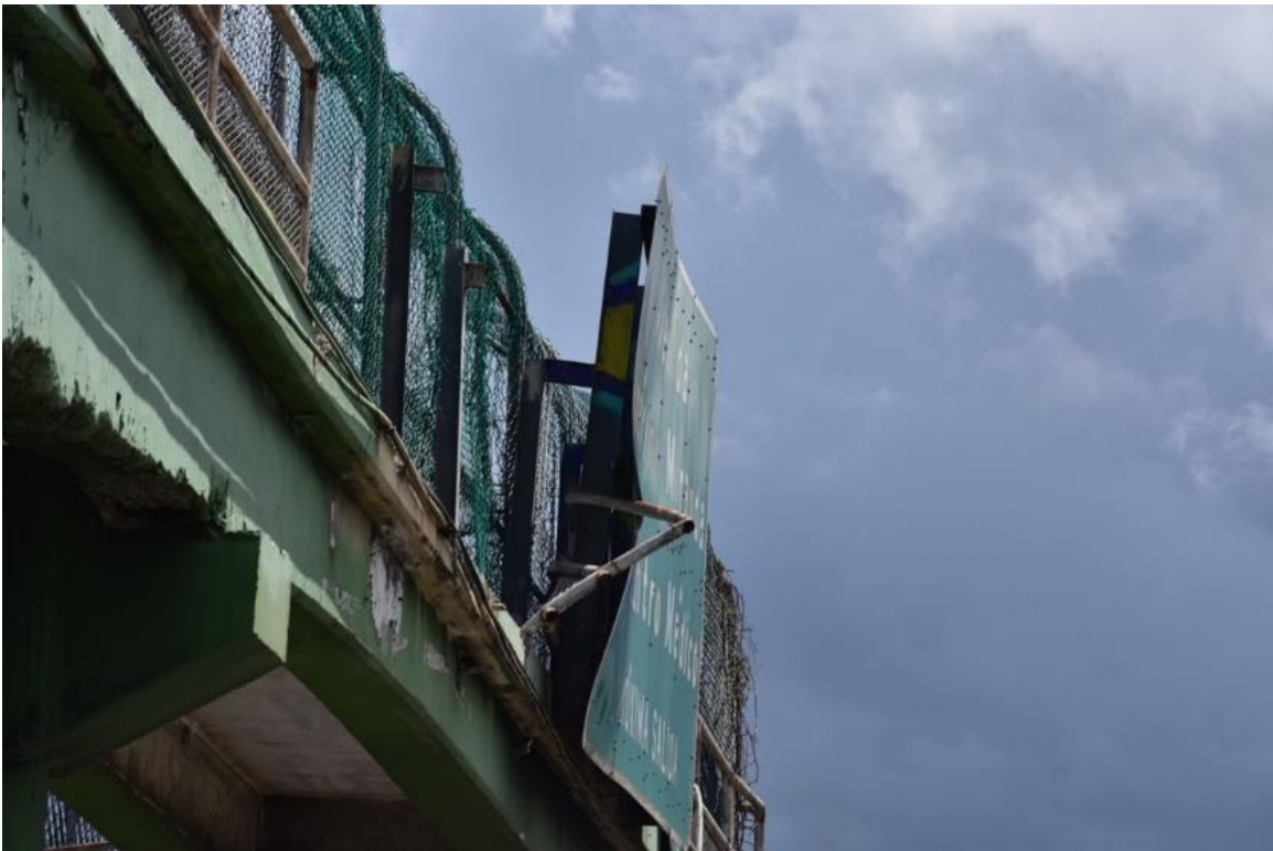
Figure 5.20: Deformed sign due to handrail bent
