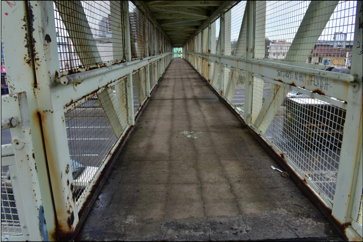
Figure 6.38: Corrosion on the superstructure of PB 2682
