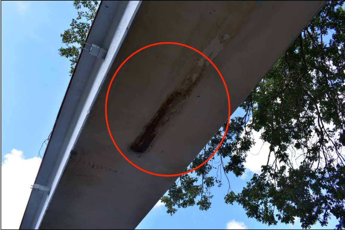
Figure 6.5: Exposed rebar on PB 0626
