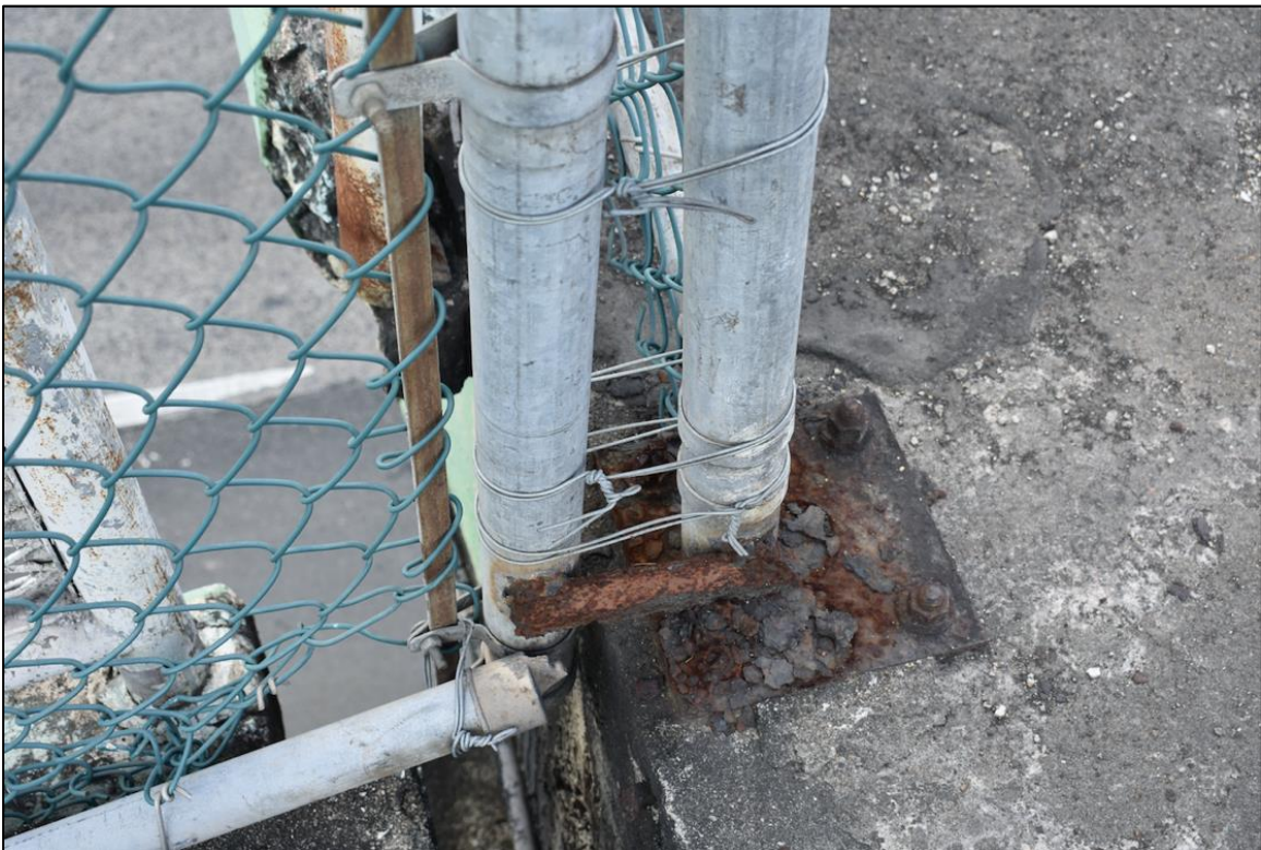
Figure 5.15: Corrosion in base support of chain-link fencing
