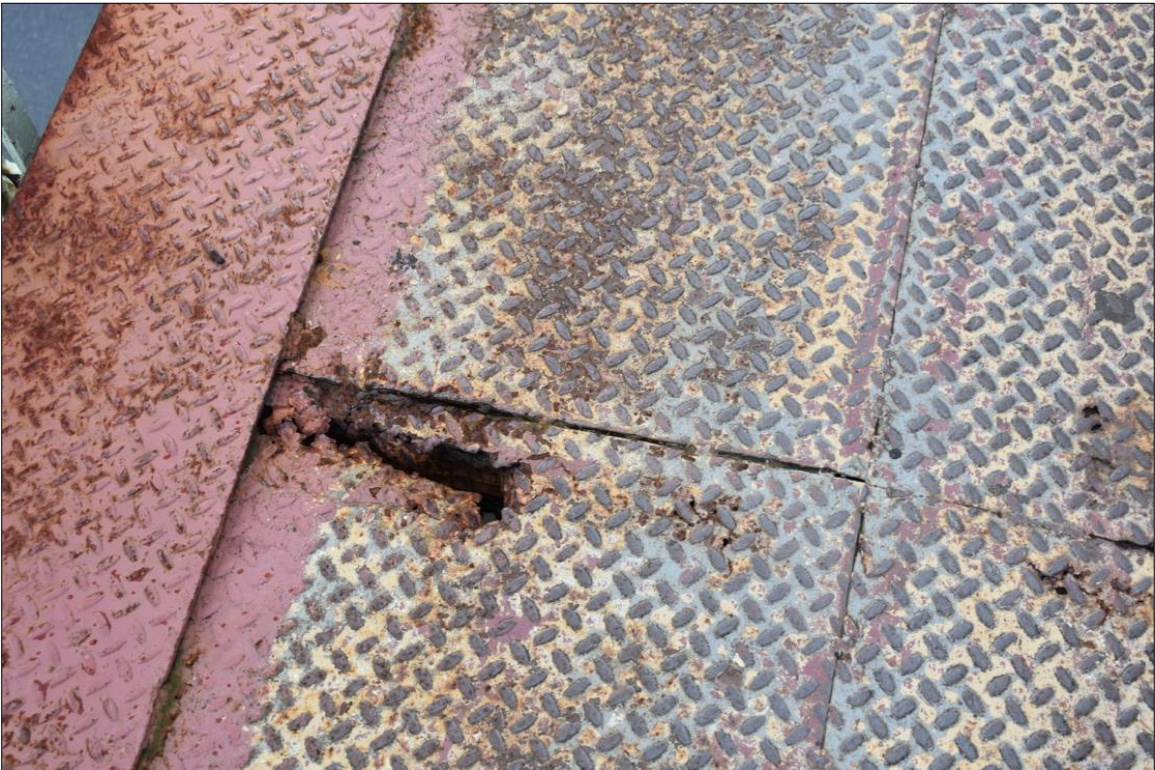
Figure 5.64: Hole in plates
