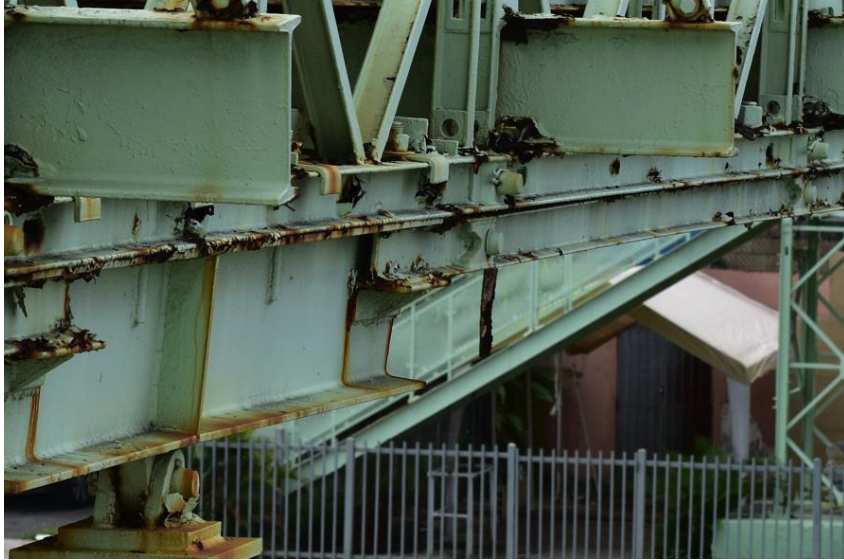
Figure 5.14: Corrosion in Floor Beams (Example 2)
