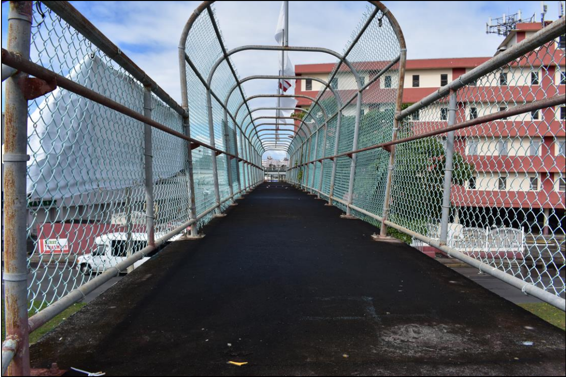
Figure 6.10: Mold and silt on PB 1095
