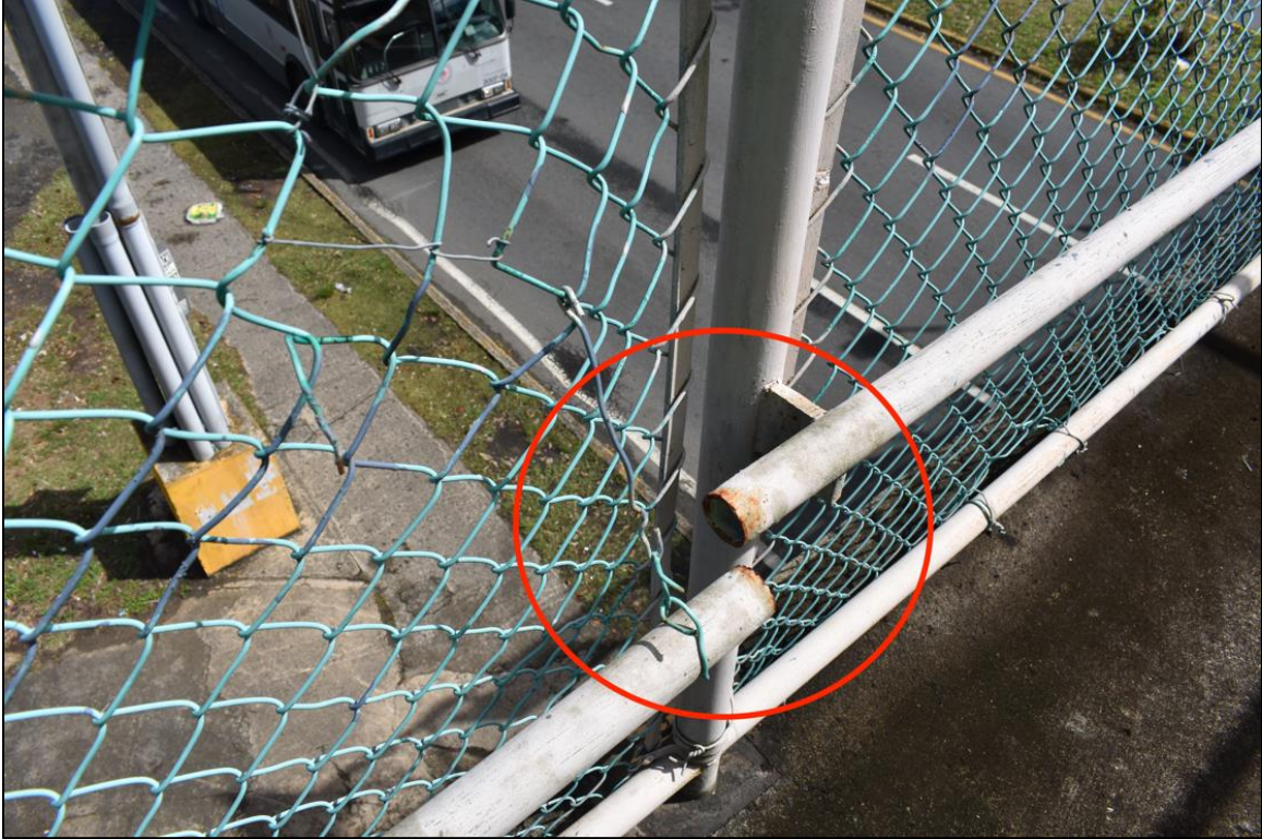
Figure 6.15: Broken railings on PB 1418
