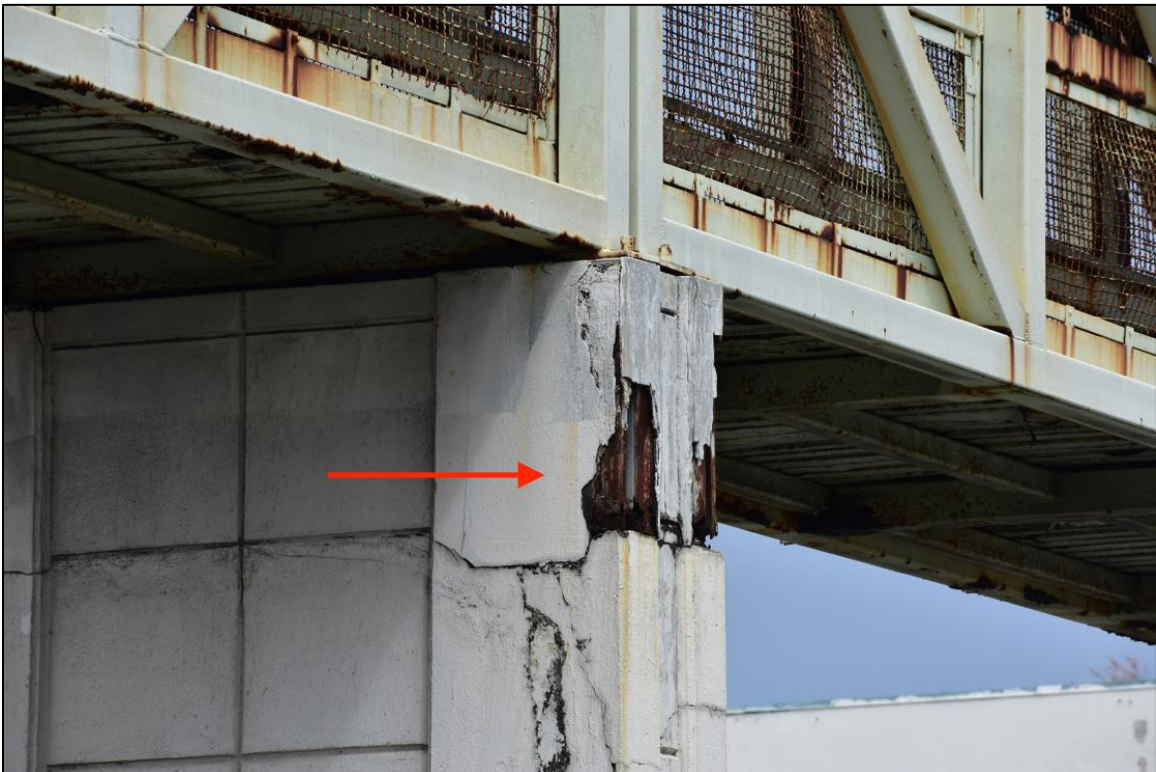
Figure 6.37: Damage to the façade and signs of corrosion on the center pier of PB 2682
