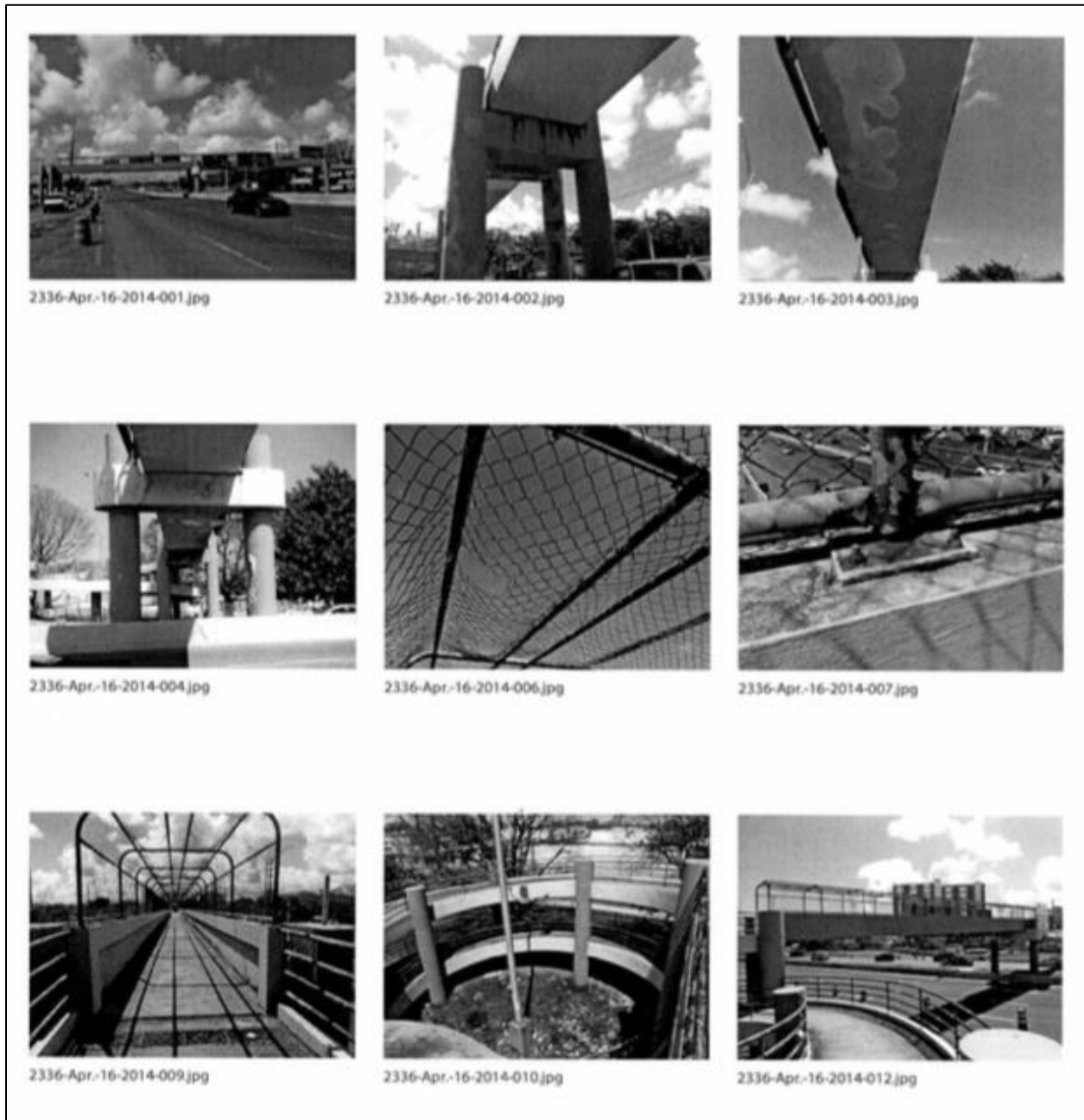
Figure 5.70: Photos of the inspection report dated April 14, 2016 (Source: PRHTA)
