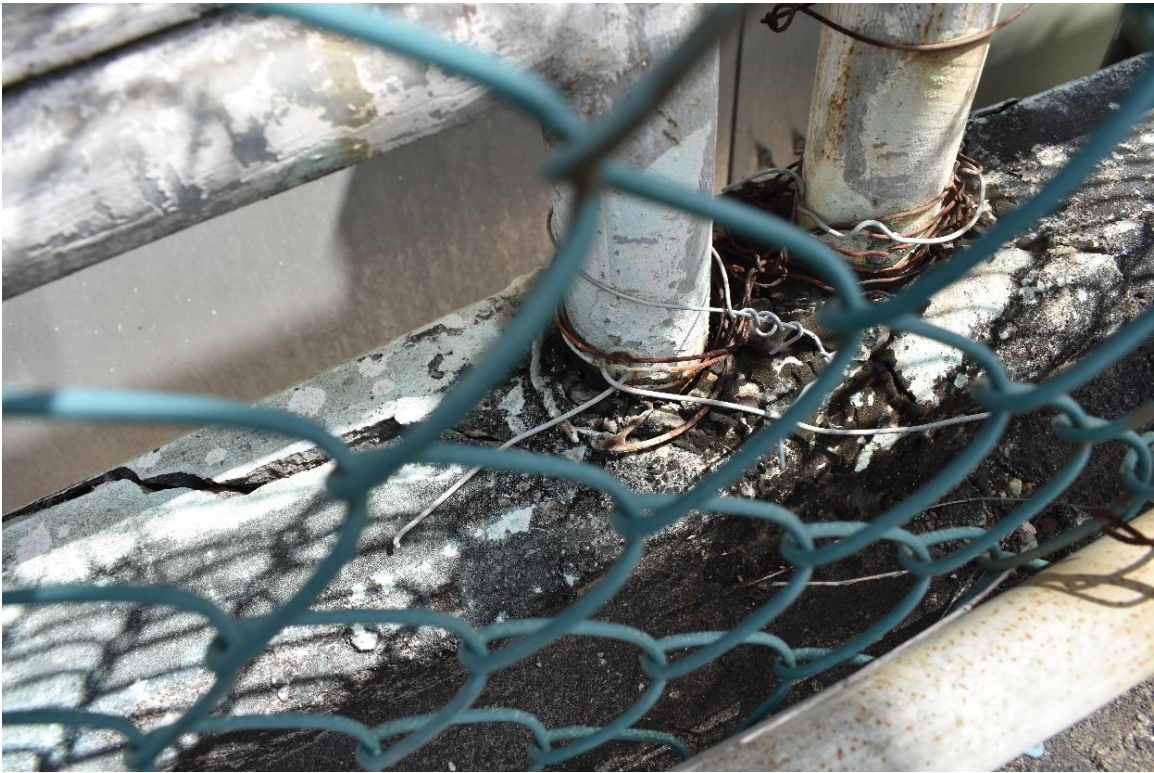
Figure 5.18: Cracks at the base of the handrail posts
