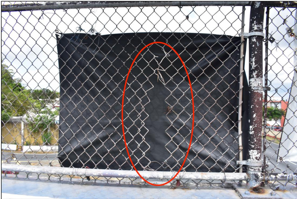
Figure 6.34: Security Fence with holes, Pedestrian Bridge 2355
