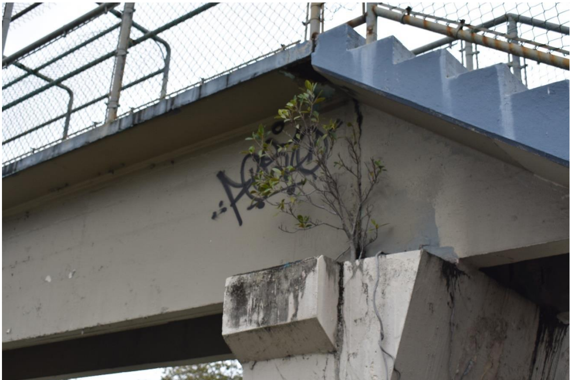
Figure 6.27: Vegetation on pier of PB 1743
