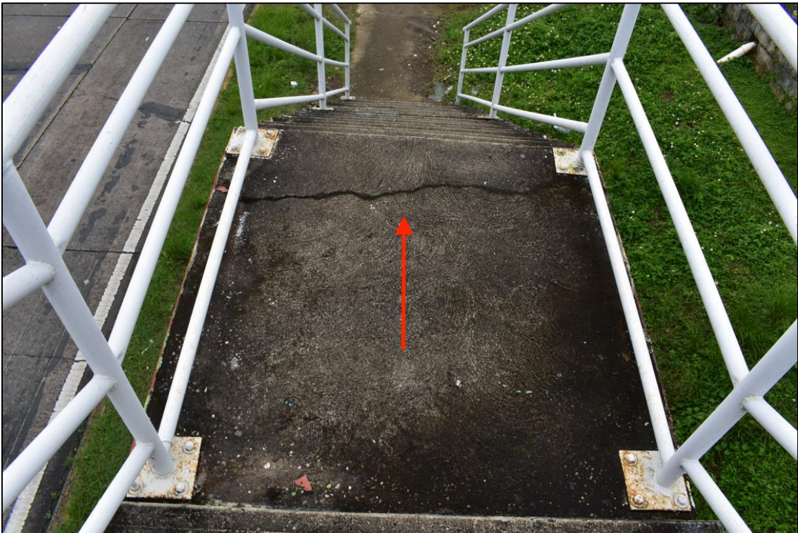
Figure 6.24: Crack on stairway of PB 1736
