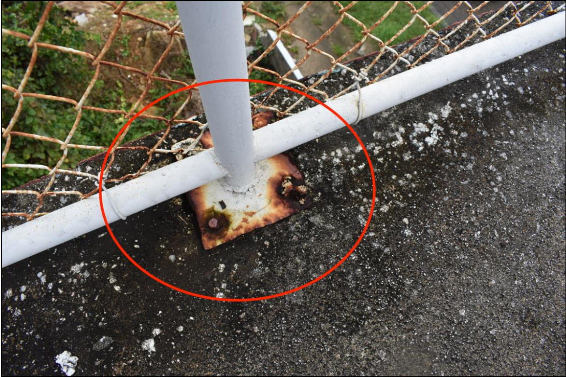
Figure 6.23: Corrosion of security fencing on PB 1736
