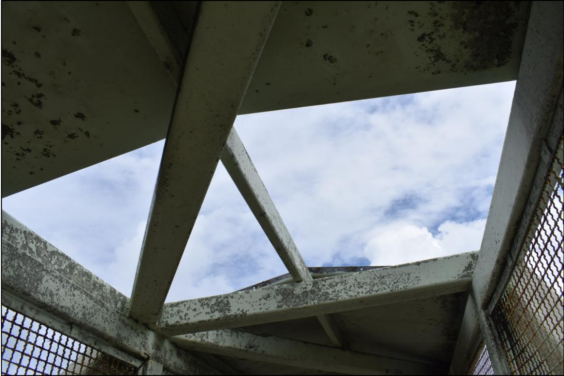
Figure 6.41: Missing roof panel on PB 2683
