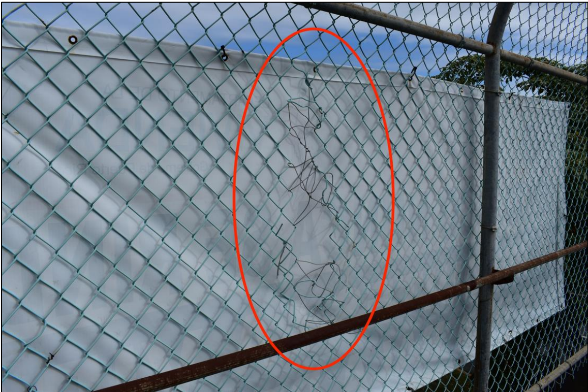
Figure 6.11: Hole in safety fence on PB 1095
