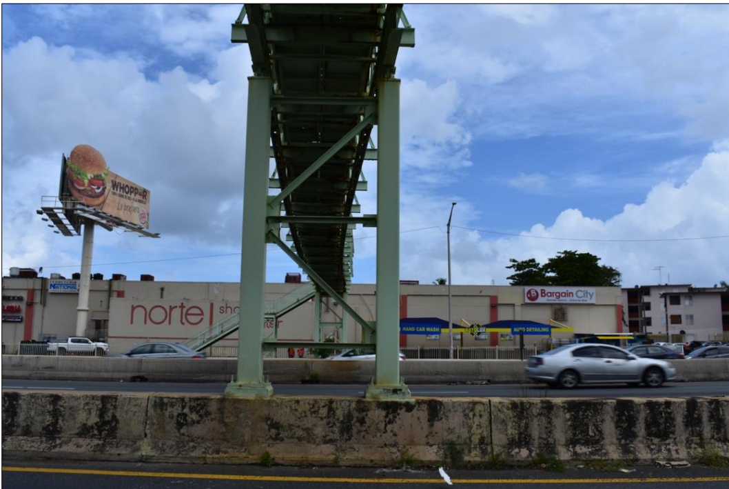
Figure 5.37: Underside of PB 1137 after Hurricane Maria (November 3, 2018)
