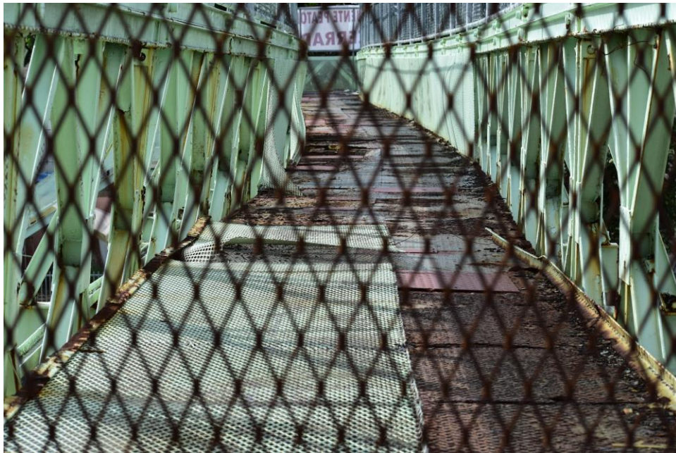
Figure 8.17: Twist of the Truss Panel
