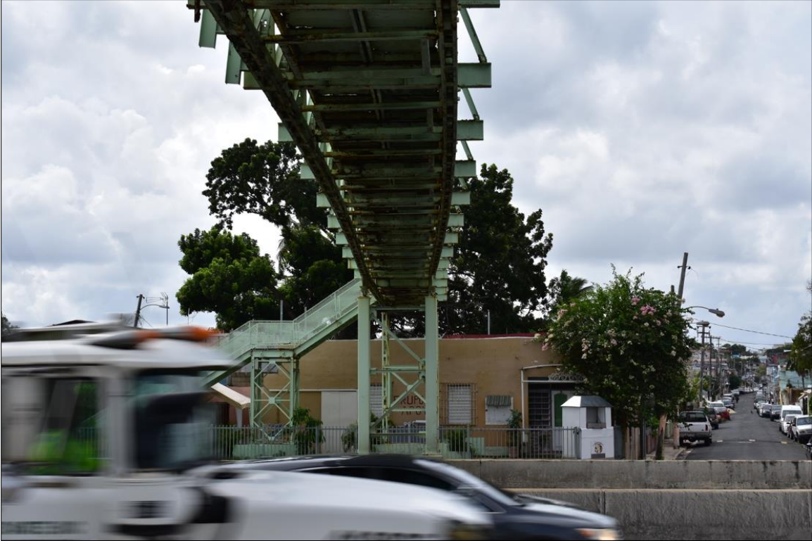
Figure 5.42: Underside view of lateral deflection
