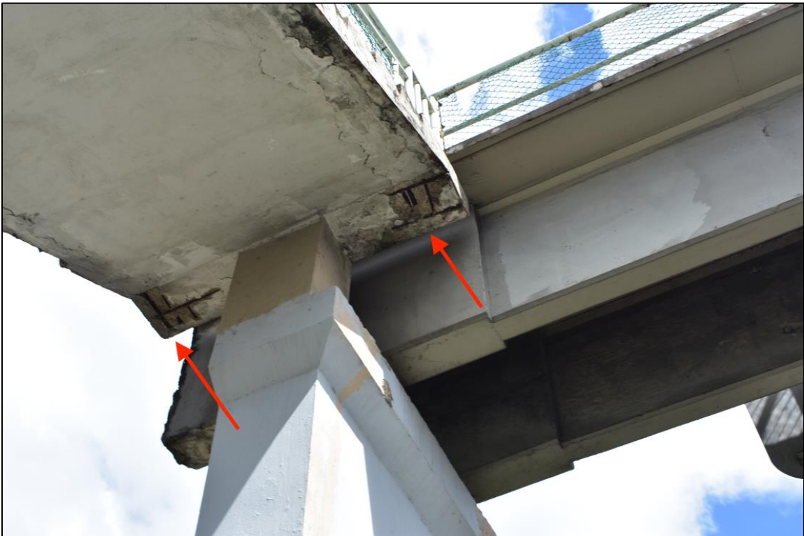
Figure 6.31: Exposed rebars on PB 2087
