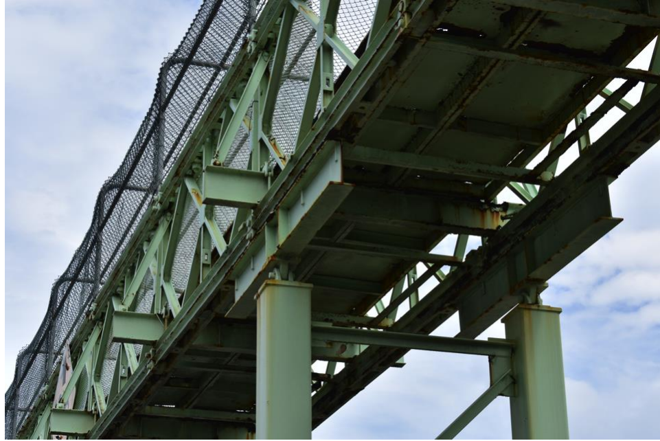
Figure 5.8: Loss of Decking due to Corrosion and Missing Bracing Elements
