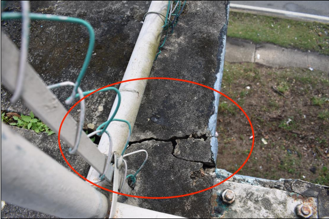
Figure 6.13: Cracks on PB 1418
