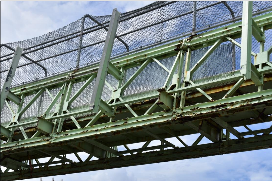
Figure 5.43: Base of the Traffic Sings
