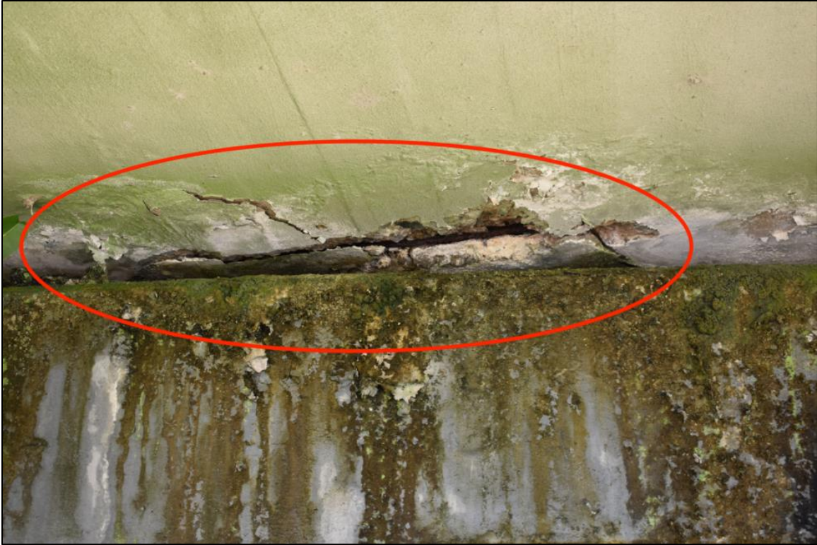
Figure 6.9: Exposed rebar on PB 0748
