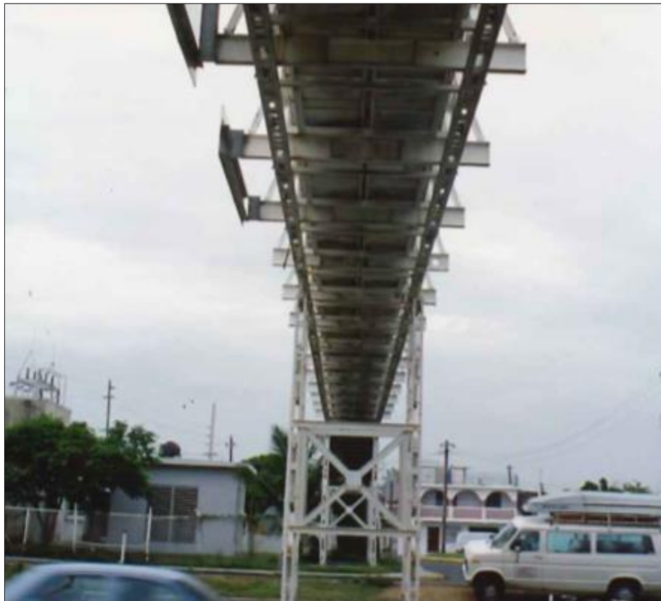
Figure 5.55: Photo of underside of PB 1307 taken on September 24, 1993 (Source: PRHTA)
