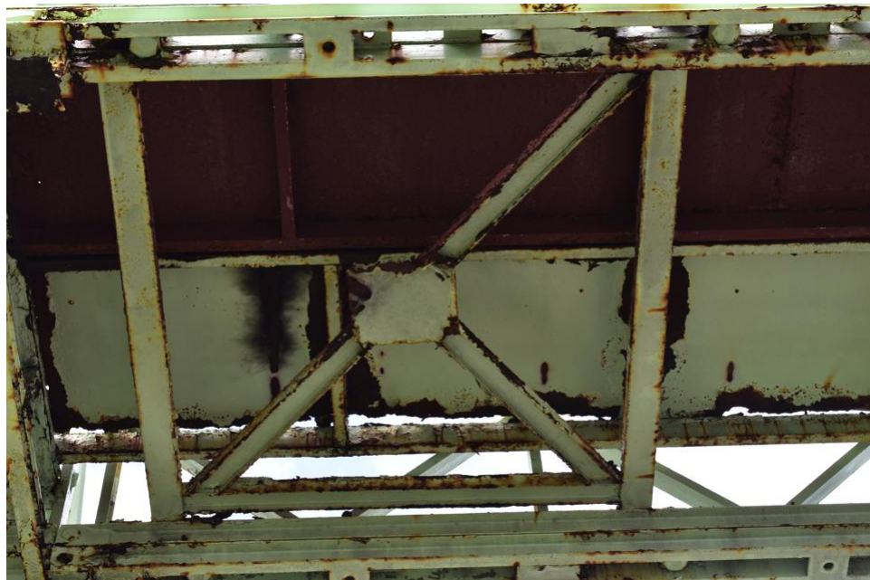
Figure 5.9: Missing Bracing Elements
