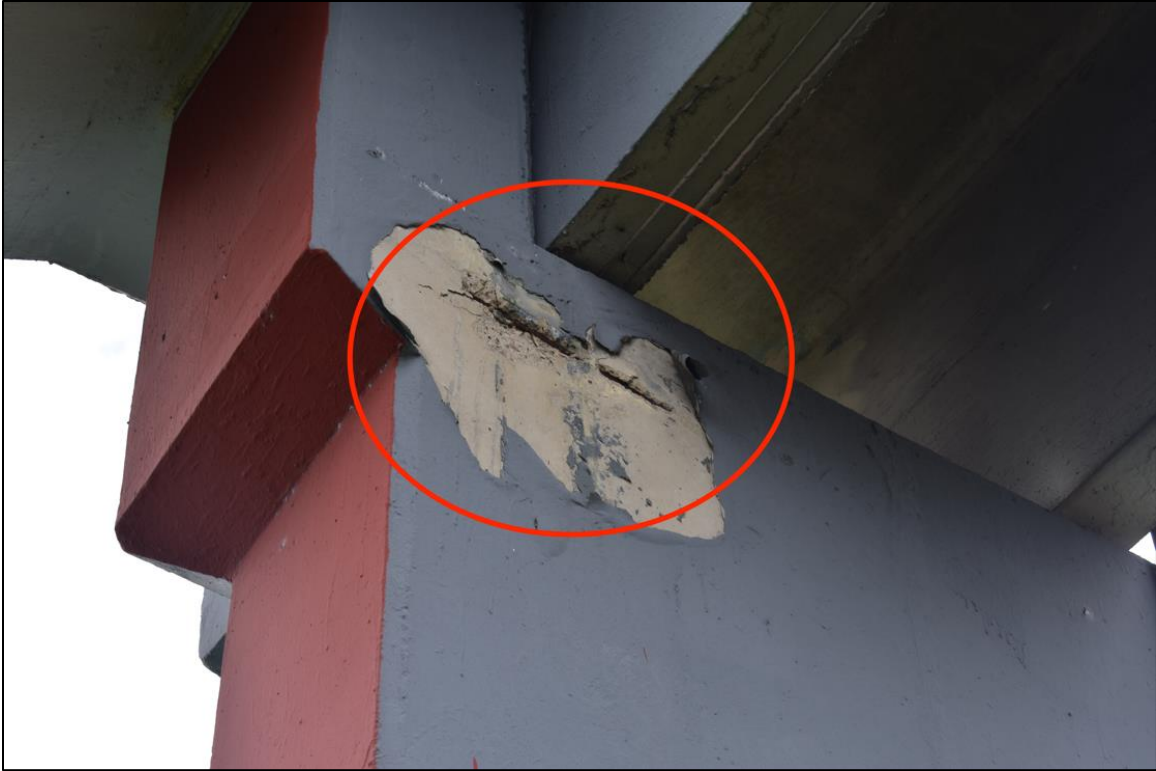
Figure 6.21: Exposed rebar on PB 1736
