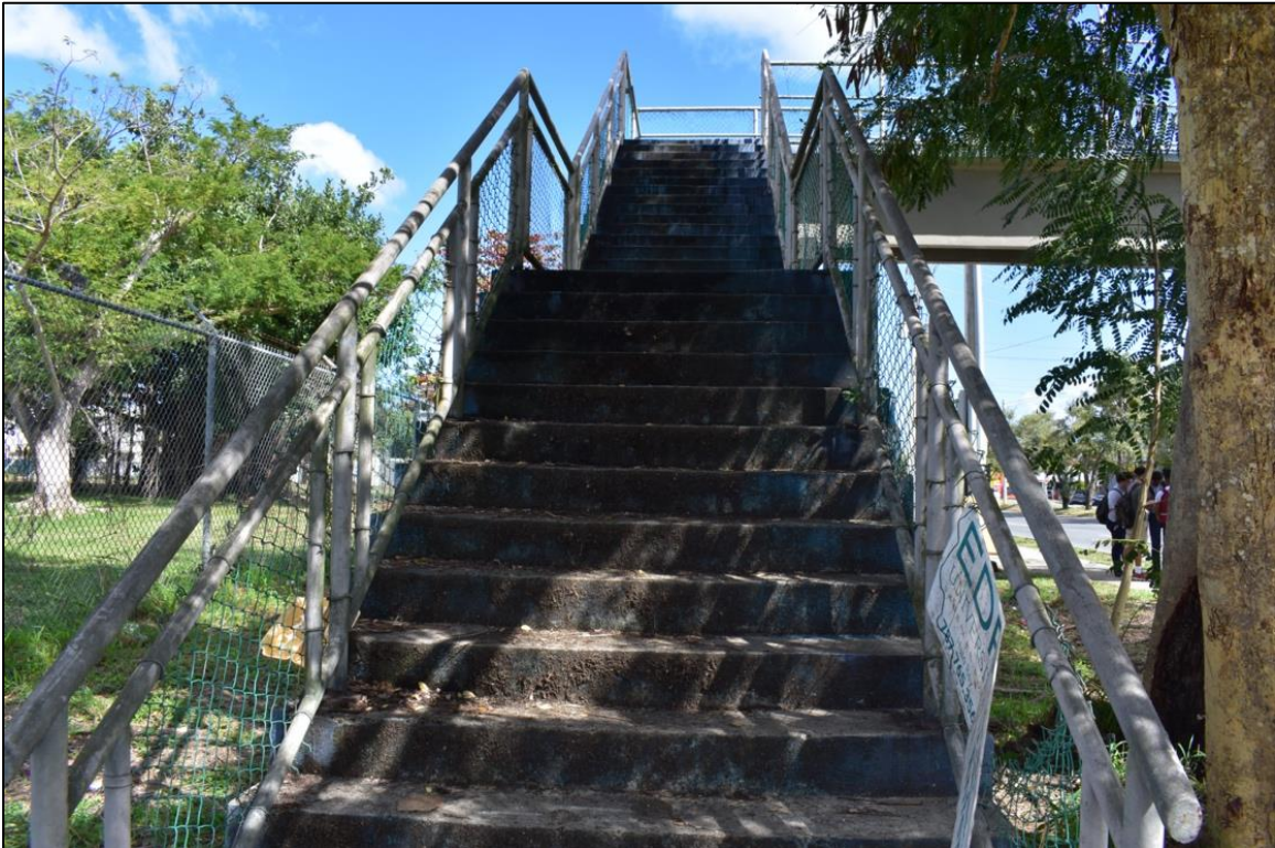
Figure 6.12: Mold on stairways of PB 1418
