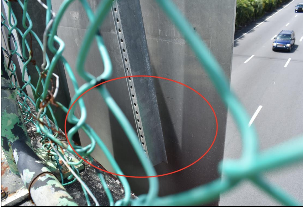
Figure 5.74: Transit sign detached from mounting assembly
