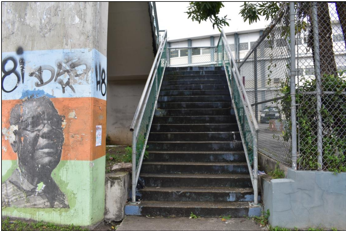
Figure 6.25: Mold and silt on stairway of PB 1743
