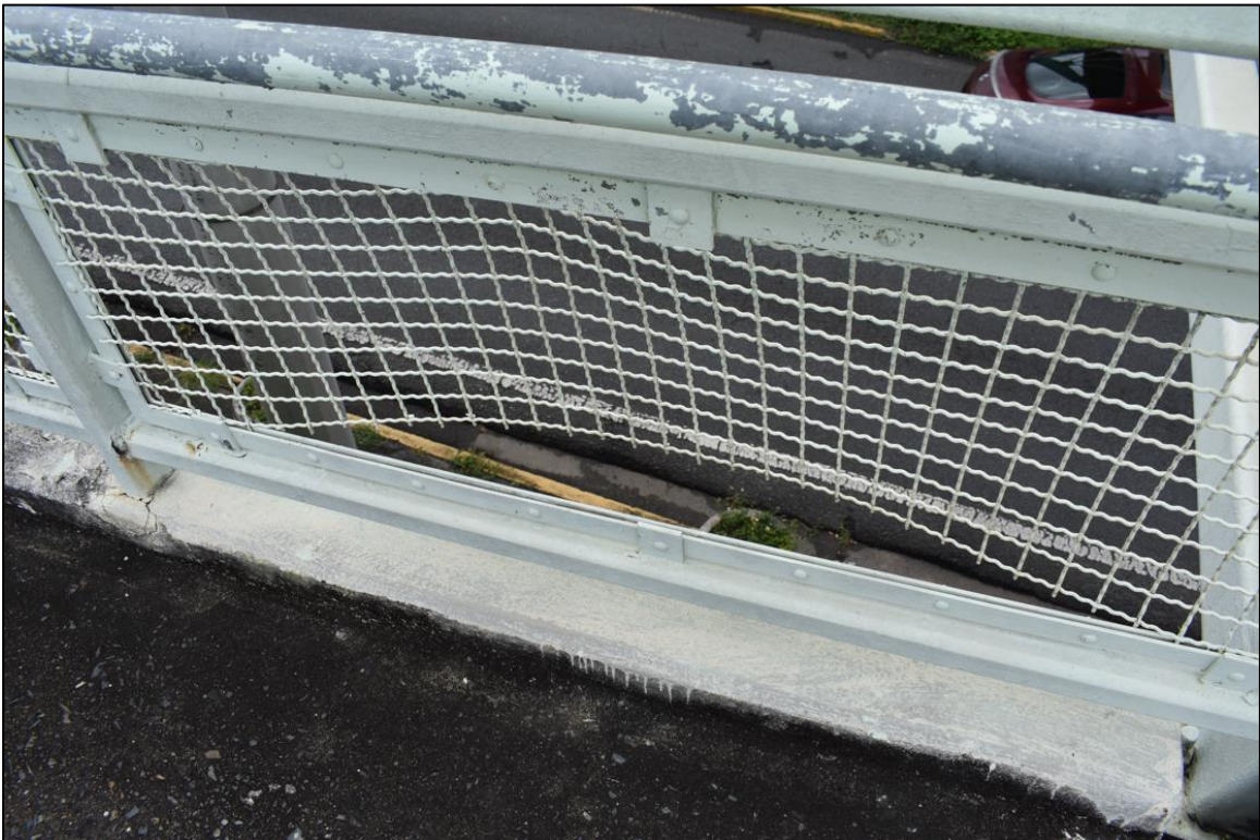
Figure 6.42: Detachment of security mesh on PB 2683
