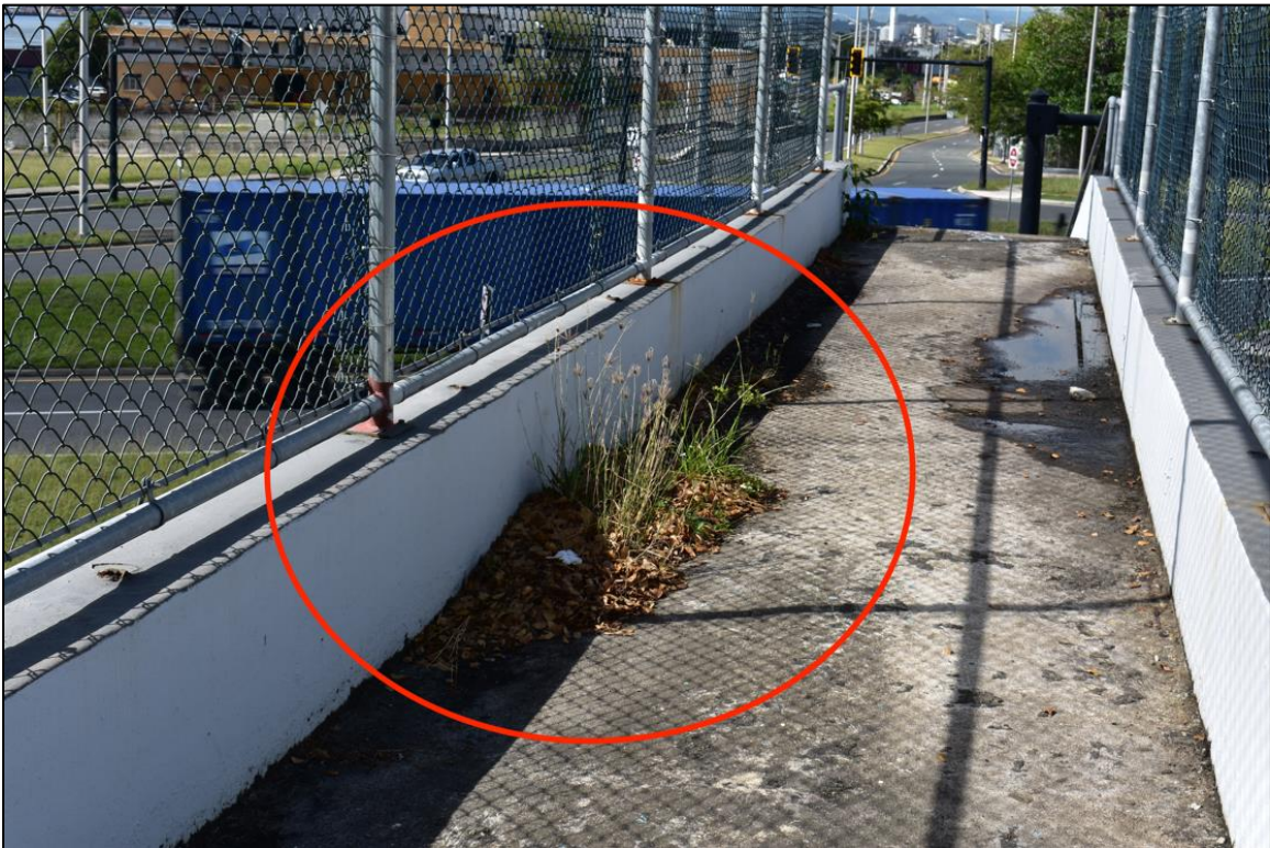
Figure 6.7: Blocked pluvial drains in PB 0745
