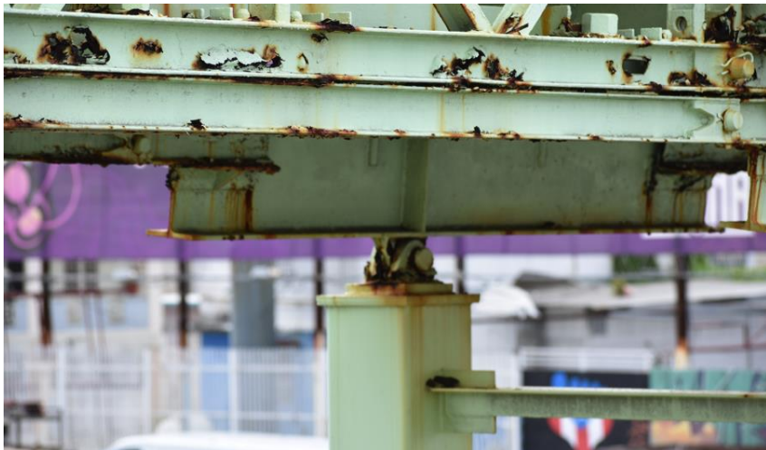
Figure 5.12: Corrosion in Truss Element (Example 3)
