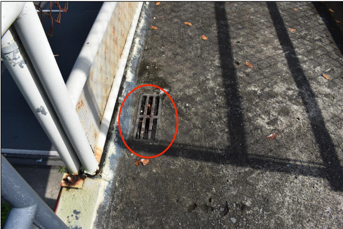
Figure 6.2: Blocked pluvial drain in PB 0626
