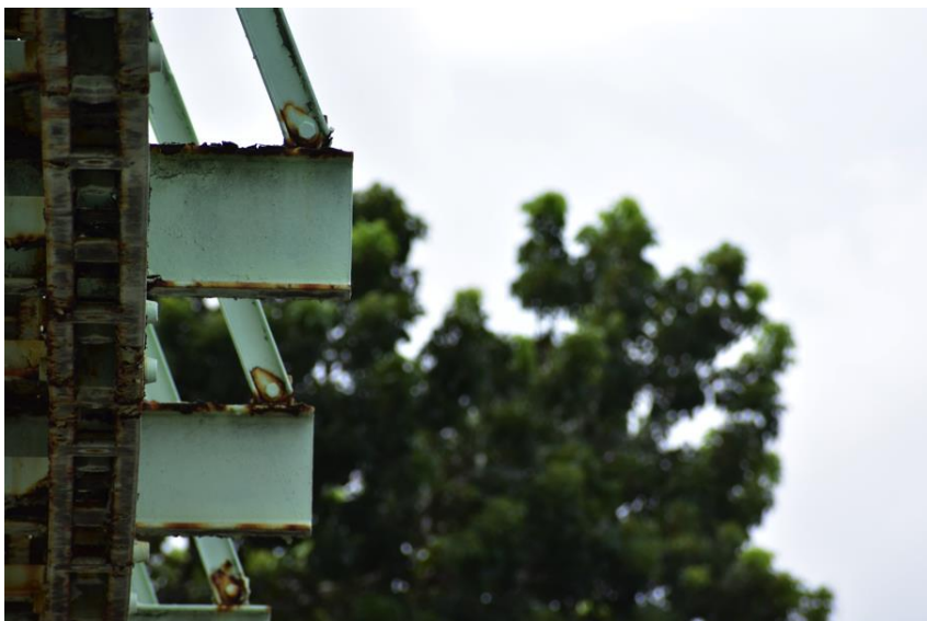
Figure 5.13: Corrosion in Floor Beams (Example 1)
