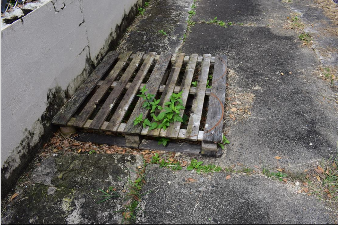
Figure 5.12: Holes in sidewalk covered with a pallet
