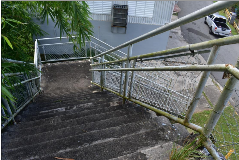
Figure 6.20: Mold and silt on PB 1513
