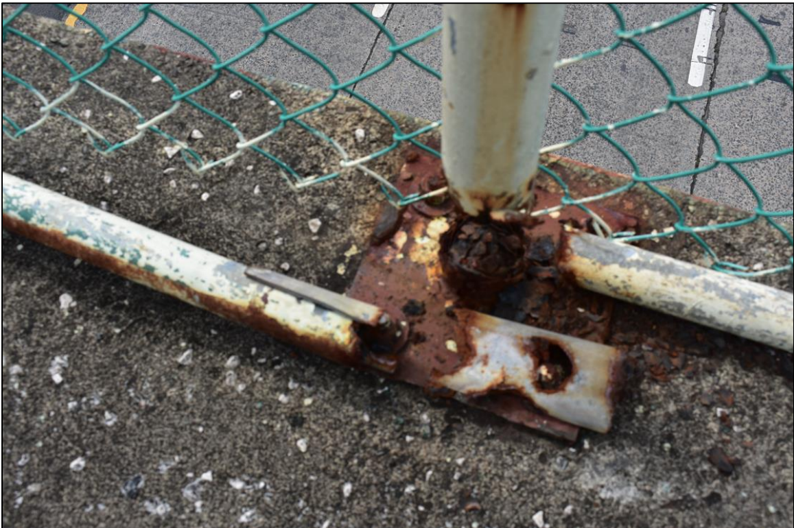
Figure 6.33: Corrosion of security fencing on PB 2087
