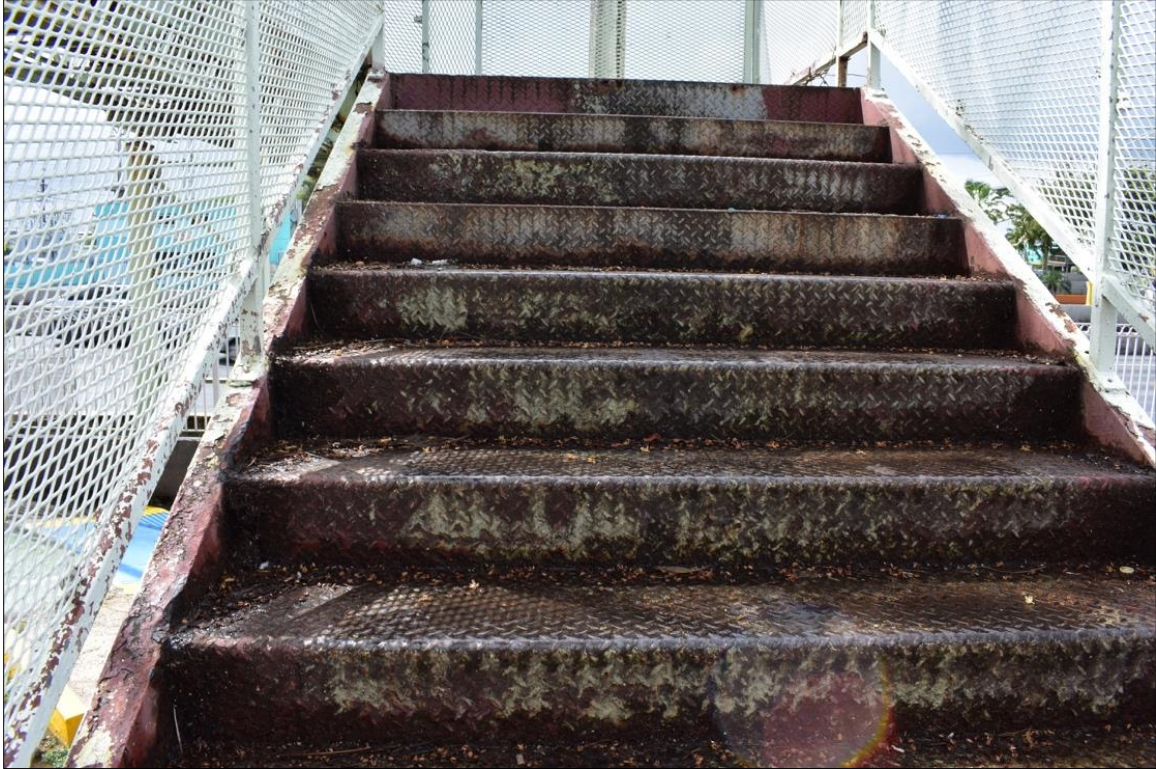
Figure 5.61: Corrosion on stairway
