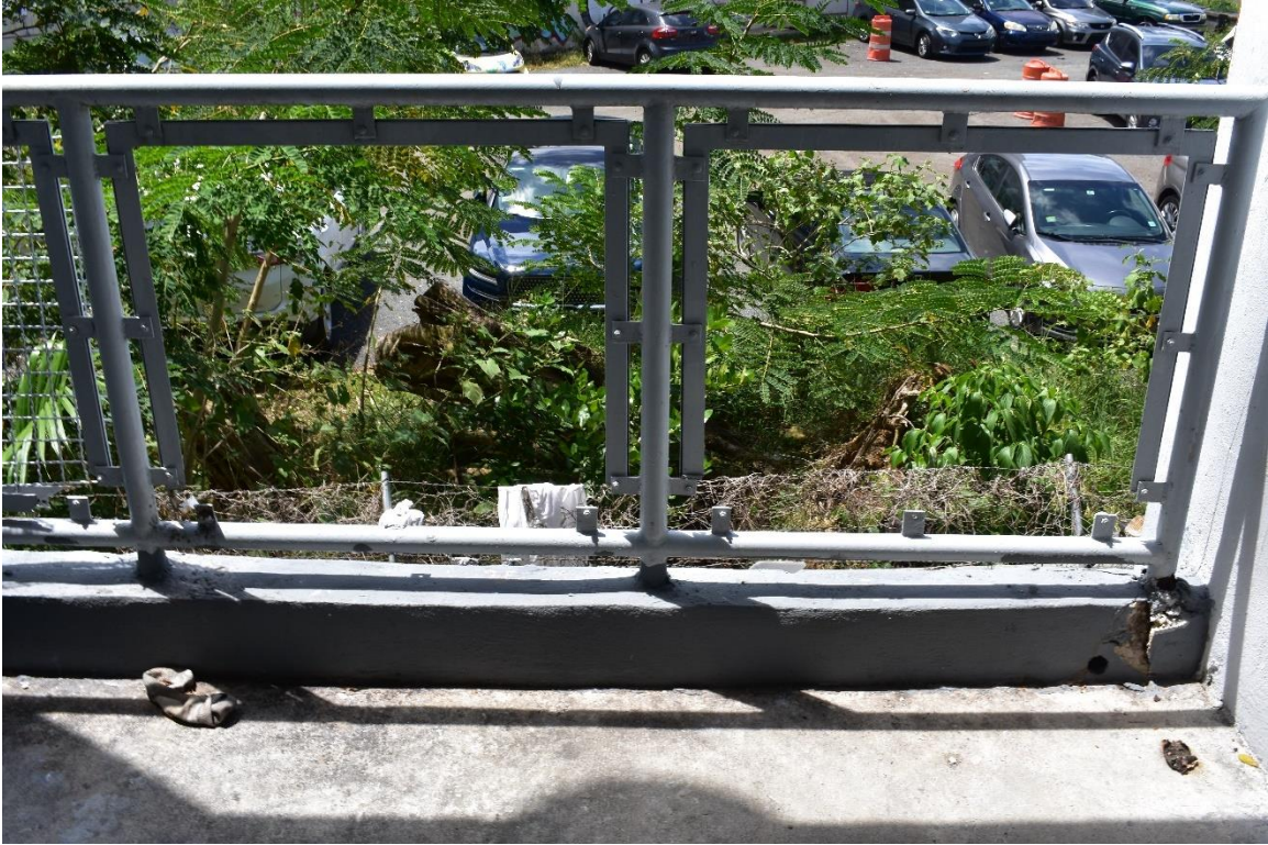
Figure 6.35: Detachment of security mesh from guardrail on PB 2566
