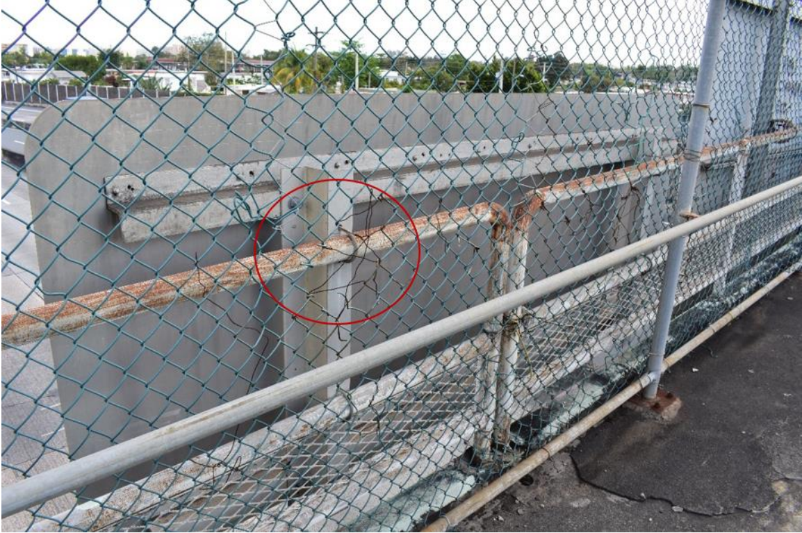
Figure 5.17: Sign mount attached to handrail
