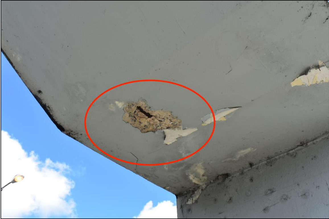
Figure 6.18: Exposed rebar on PB 1478
