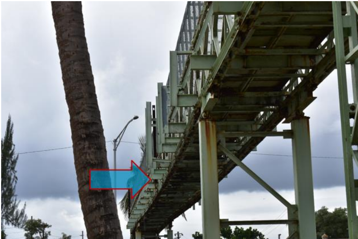
Figure 5.65: Lateral deflection at mounting assembly location
